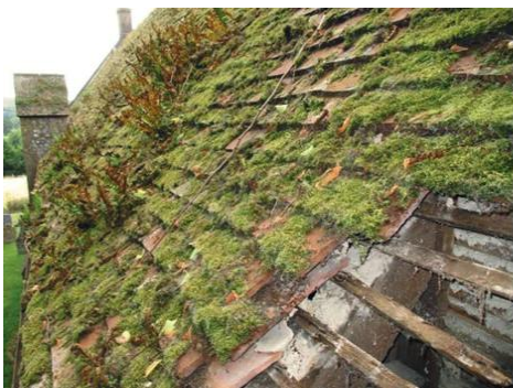
Heavy build up of moss and bracken
