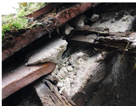
Tiles bedded on lime Rotting battens
