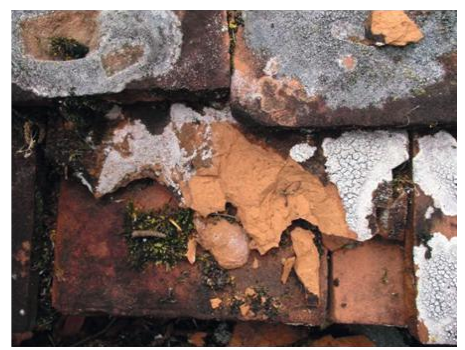
Delamination of tiles
