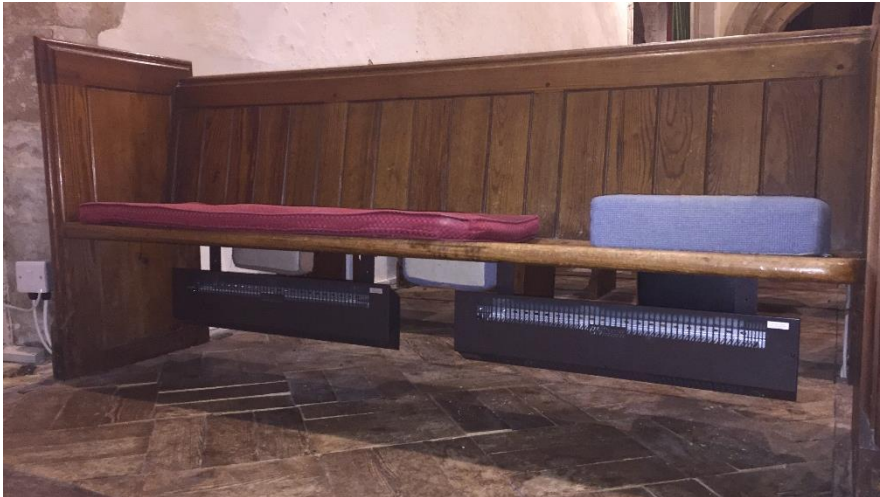
Brown BN Thermic 650W under pew heaters fixed to underside of pew seats for pews which have no solid backs.
