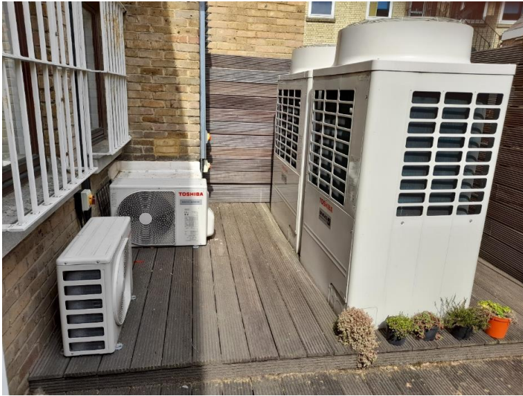
Examples of air source heat pump external units, comprising of three smaller 3kW units and two larger 10kW units.
