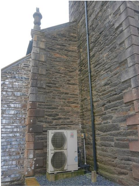
A monobloc air source heat pump at St Anne's Church, Ings, Cumbria - Photo credit - Historic England/Max Fordham LLP
