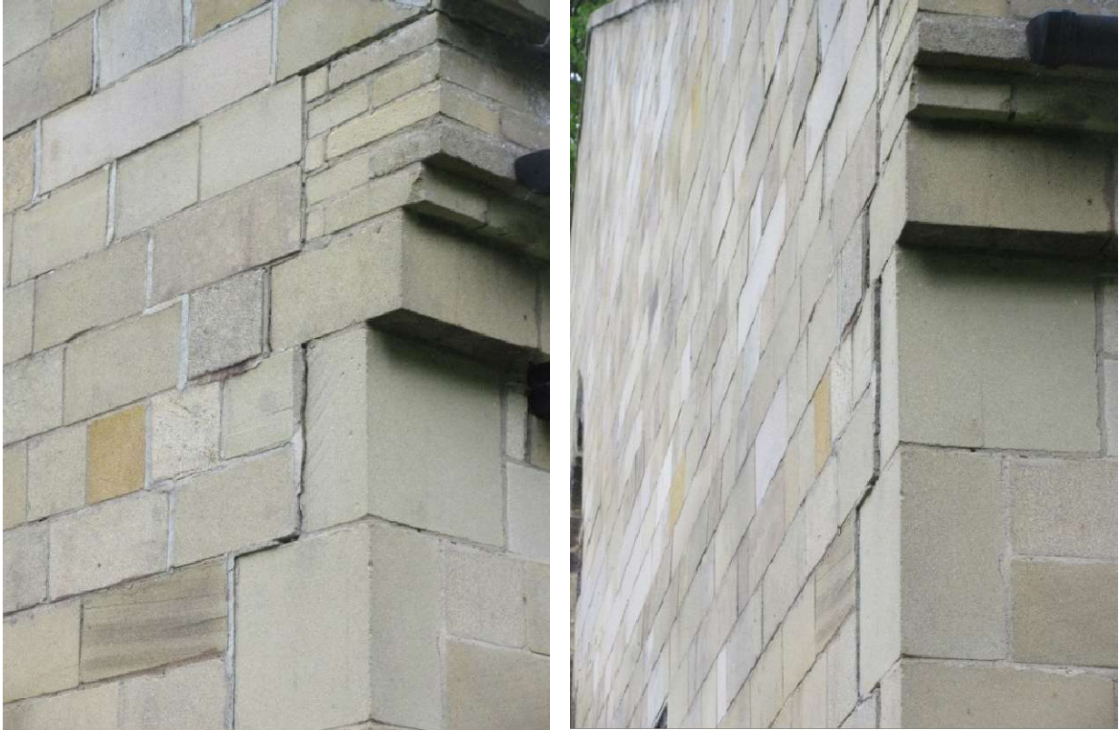
Paragraph 30 – signs of separation of stone cladding at the SW corner
