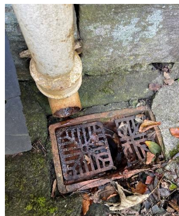
Figure 6- broken gully to N Nave
