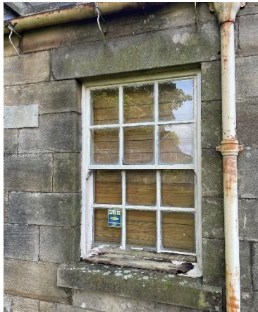
Figure 11- NE weathered window
