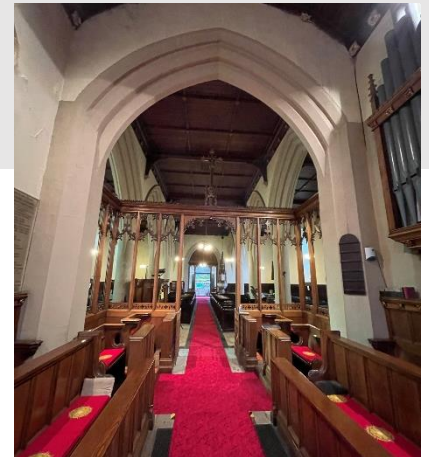
Figure 16- Chancel Arch with staining
