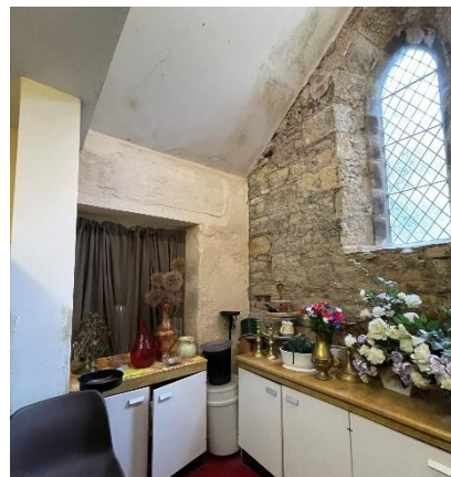
Figure 17 - Damp wall to NE vestry
