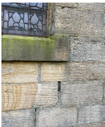
Figure 7- Crack to NE window
