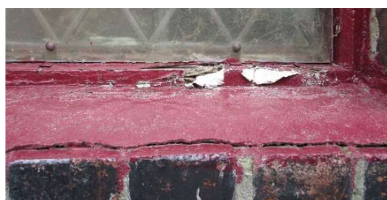
decay in a Nave W cill
