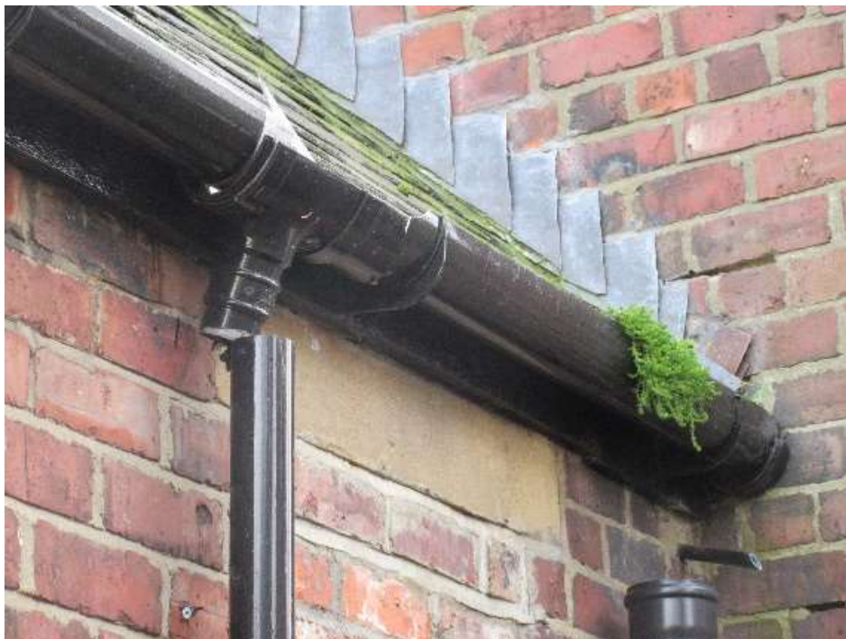
W side of offshot – outlet disconnected from gutter and pipe and gutter blocked
