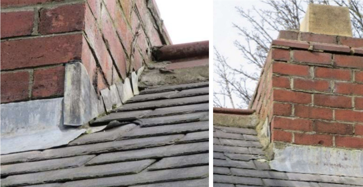
Lead cover flashings missing from both S sides of the chimney
