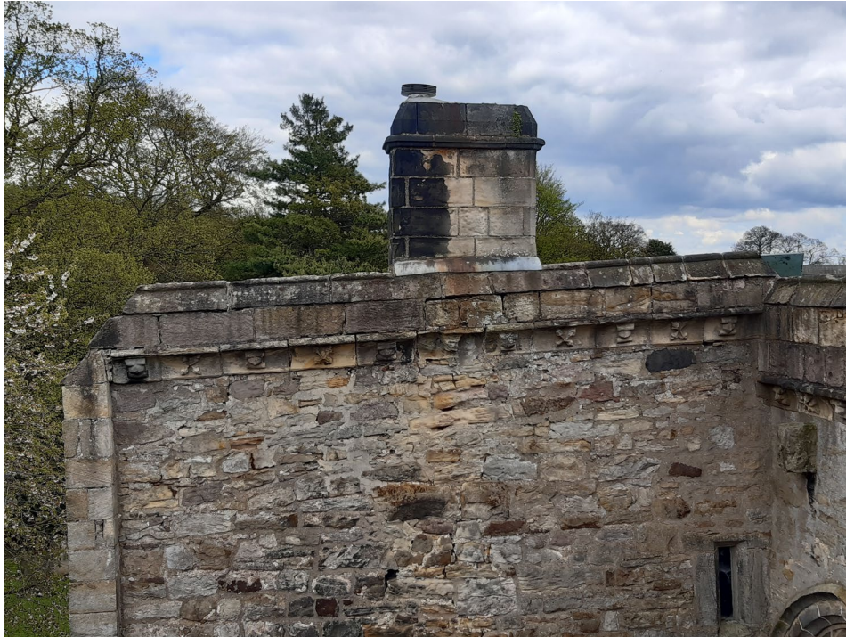
North Vestry, west facing wall showing extensive erosion and missing mortar.
