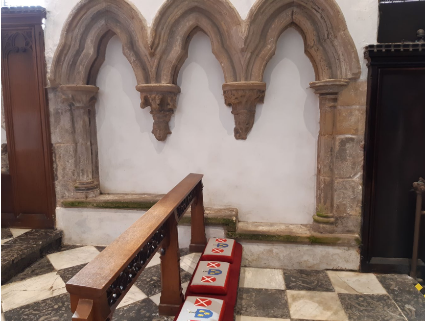
The sedilia, with low level damp mould.
