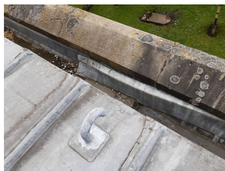
North Aisle, loose lead flashing
