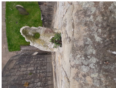
South Aisle roof drainage – ancient gargoyle with blocked outlet from downpipe
