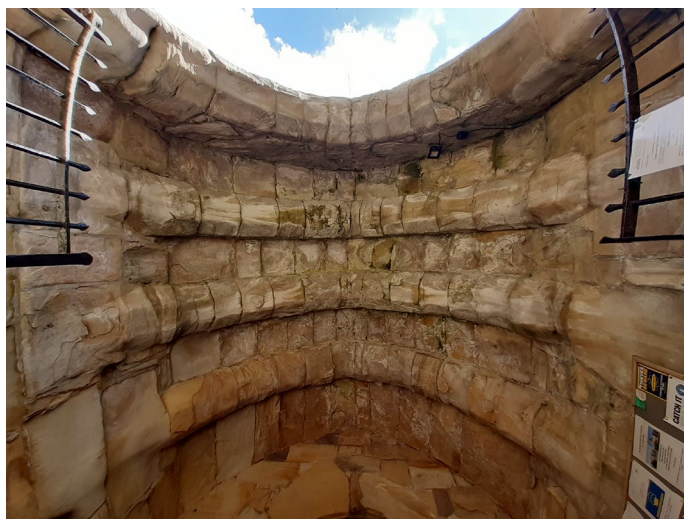
Inside the South Porch, showing damaged stonework to the vault.
