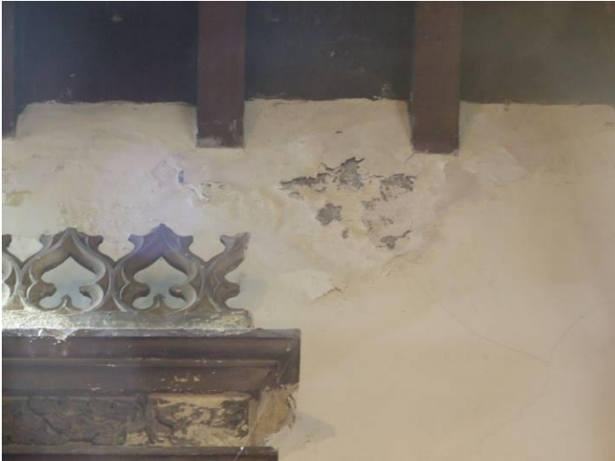
P6 (8800): Efflorescence to chancel north wall, above monument
