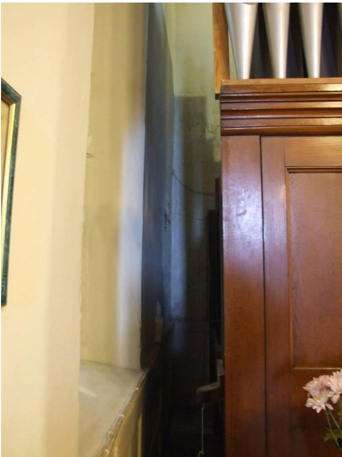
P2 (8798): Efflorescence to north chancel arch wall, behind organ
