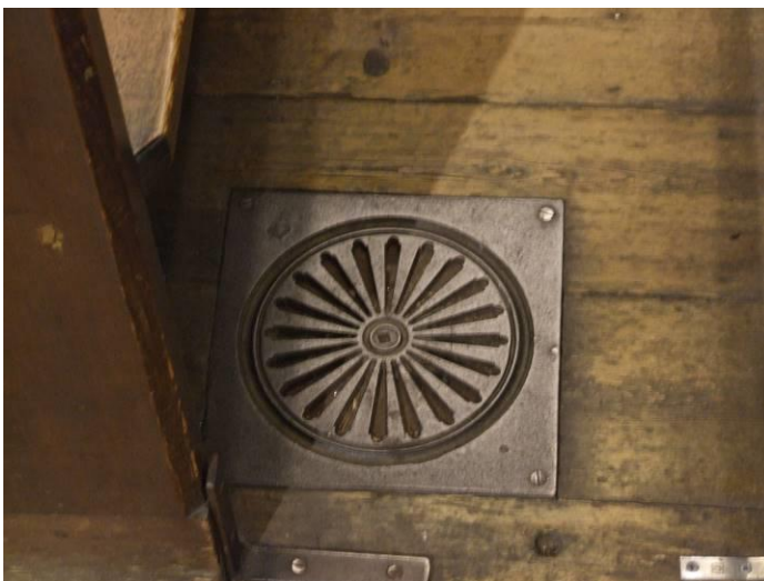
P13 (8834): Redundant floor heating outlet
