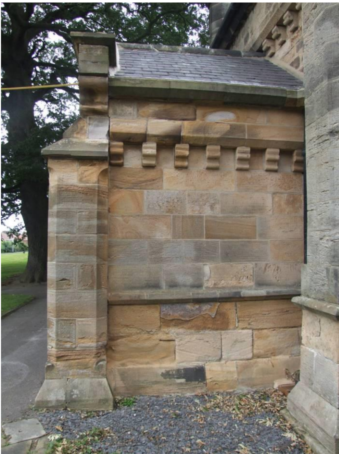
P24 (8859): South porch, low level stone face loss
