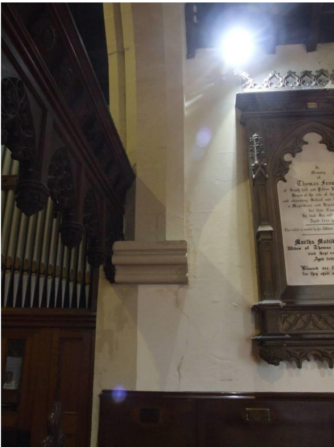
P5 (8799): Efflorescence at northern side of chancel arch, chancel north wall
