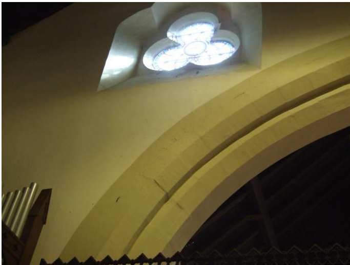
P4 (8797): Chancel arch, slight stone displacement
