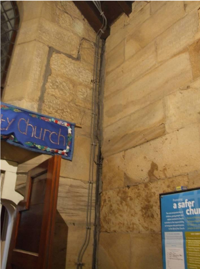
P21 (8856): Movement cracking between south porch interior and nave
