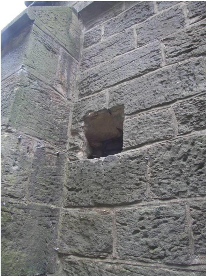
P31 (8880): Stone removal, to be rectified
