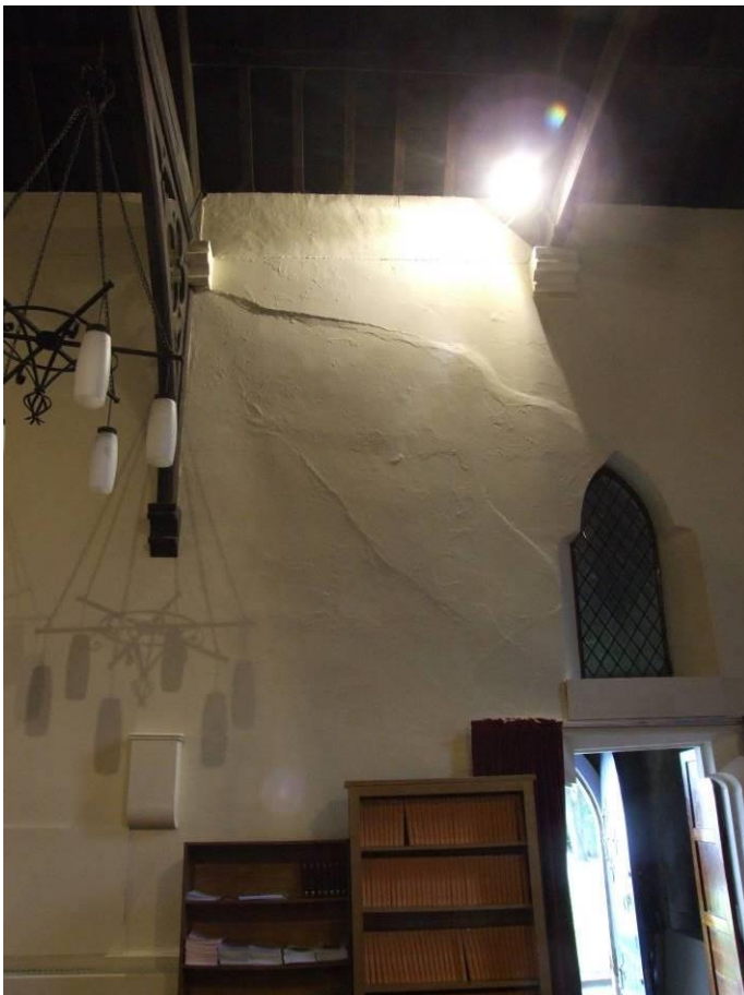
P10 (8817): Historic cracking, nave wall, south side above porch door (may relate to former organ loft position)
