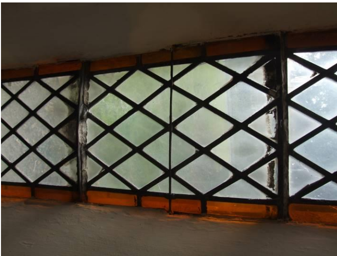
P8 (8803): Chancel south side window, leading bowed inwards
