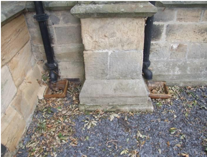
P26 (8861): Surface water gullies ahead of leaf fall
