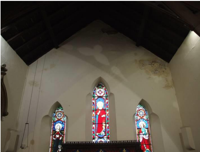
P7 (8801): High level efflorescence to chancel east wall, south side
