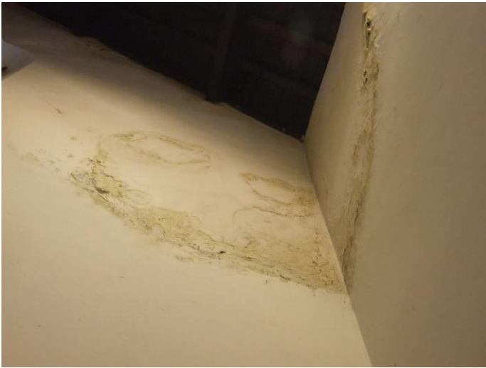
P3 (8796): Historic water staining to Nave south wall/chancel arch wall
