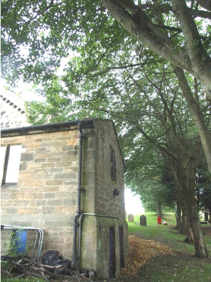
P30 (8877): Tree proximity, north side
