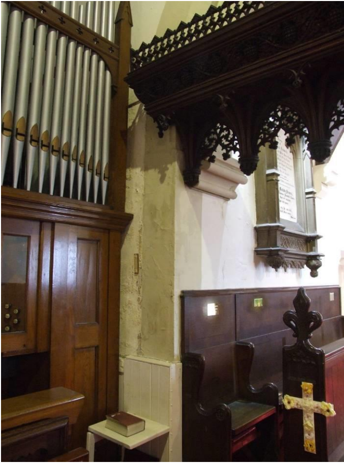
P1 (8795): Efflorescence at northern side of chancel arch
