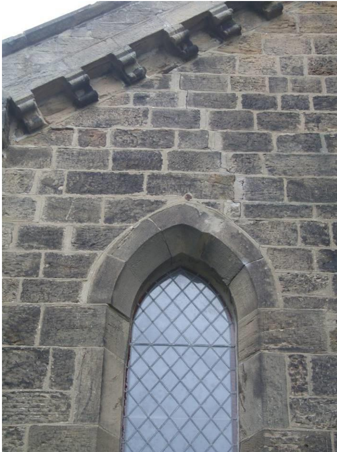
P28 (8867): Historic cracking, west end
