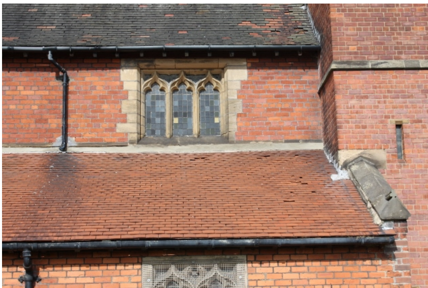
Missing roof tiles – see para 1.1
