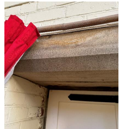
Figure 17 - crack to lintel (10.4.3)
