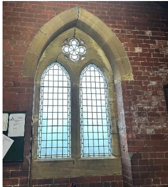
Figure 33 – cracking to E lancet
