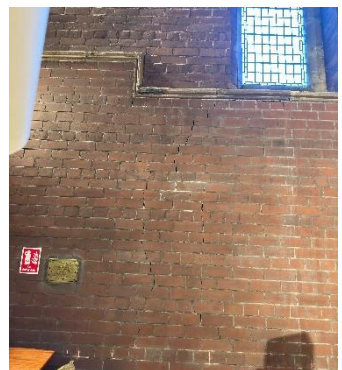
Figure 31 – cracking to N
