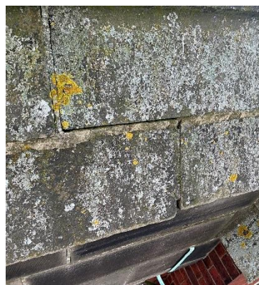
Figure 2 - Step in E side from above
