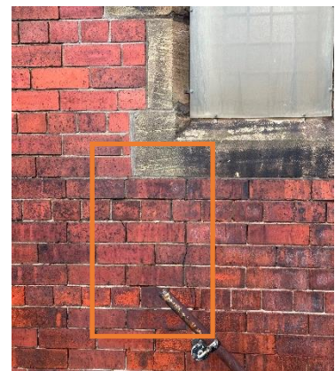
Figure 12 - crack to E Vestry window
