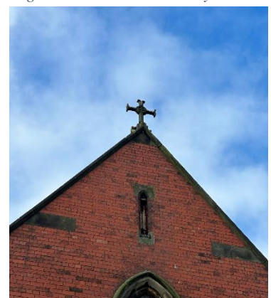
Figure 13 – E gable open joints
