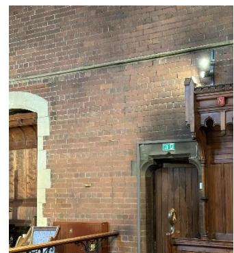
Figure 32 – cracking to S
