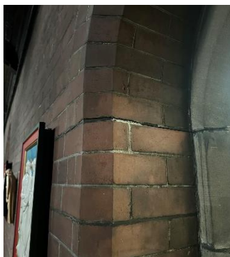
Figure 23 – crack to LHS of E
