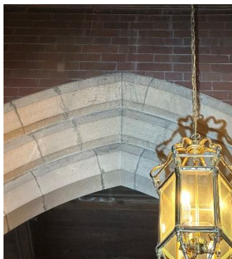
Figure 26 – crack to apex
