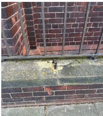
Figure 37 – cracking to W wall
