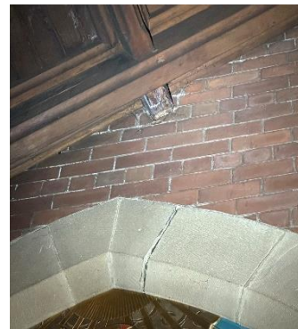
Figure 25 – purlin and crack to lady chapel
