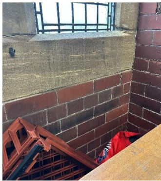
Figure 34 – below cill E wall
