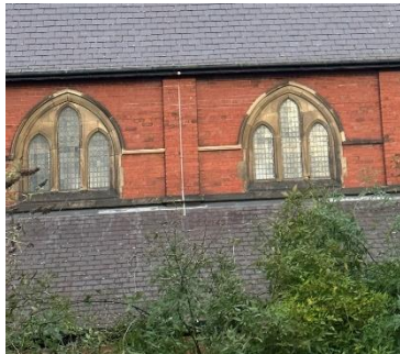
Figure 10 - erosion to mullions
