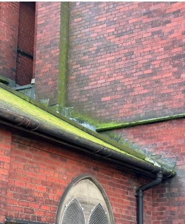
Figure 8 – Staining to N Aisle
