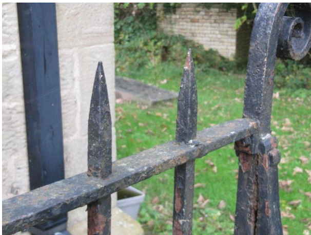
Sharp spikes to railings around the boiler house steps
