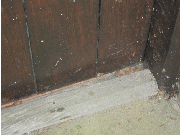
Loose threshold/weather board to vestry door
