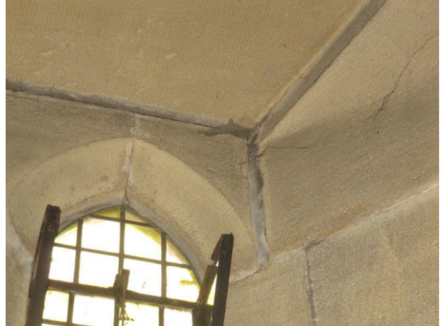
Cracking reopening to reveal of Nave windows
