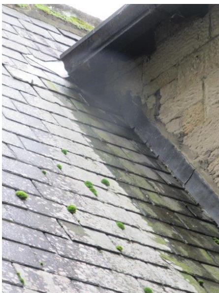
Dampness on the vestry roof from the gutter/roof over
