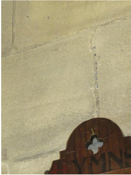
Holes left in joints from previous fixings to hymn board
