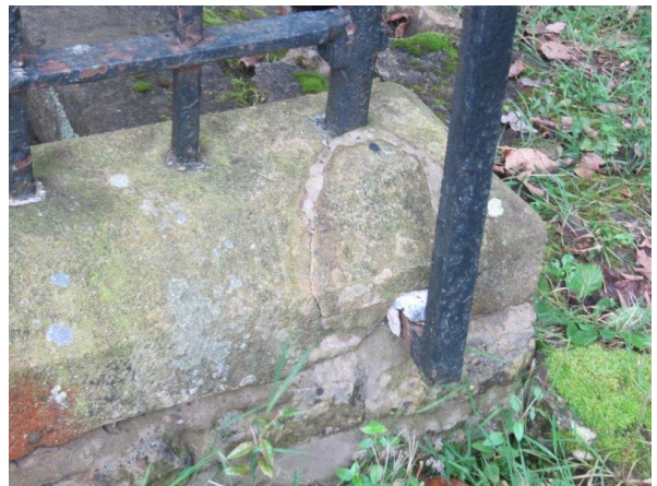
Previous mortar repair in the same area
