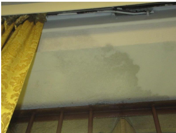
Damp staining over Vestry window
