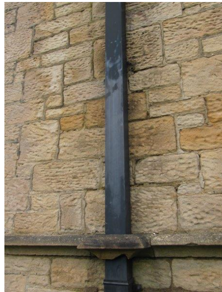
Open/hungry joints behind a downpipe on the South elevation
