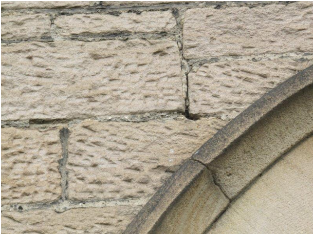
Open joints on the South Elevation
