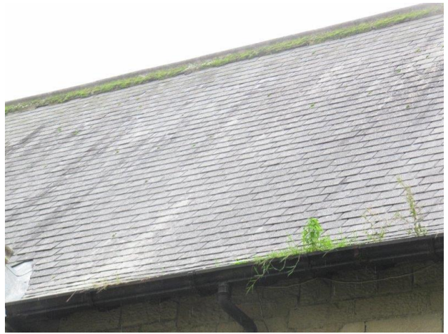
Vegetation to northern gutters
