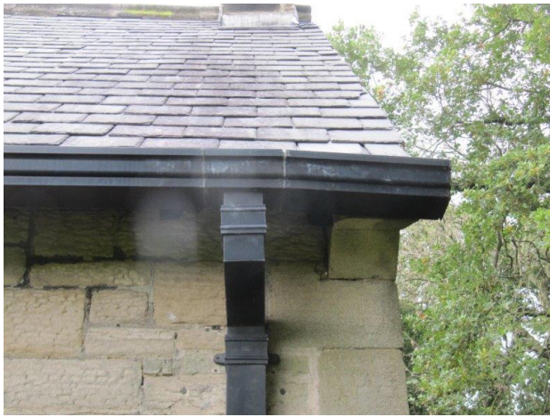
North end of the vestry gutter is poorly supported
