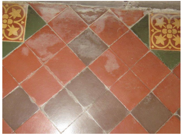
Salts/discolouration to tiles near the altar dais
