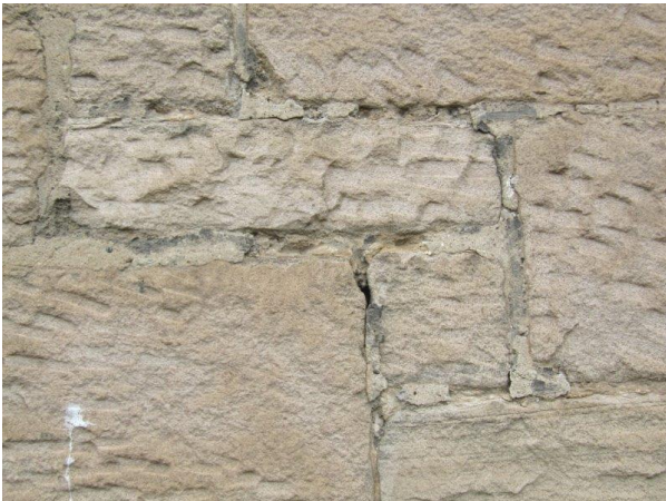
Typical issues with failing mortar
