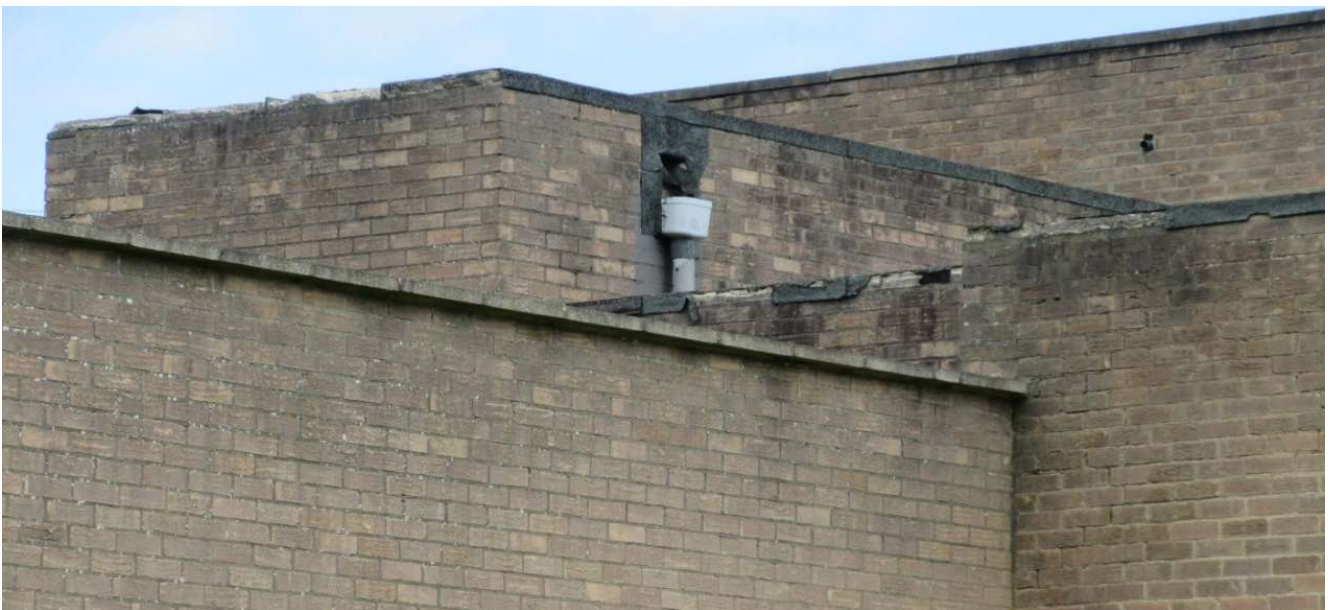
Detail of copings and parapets from the park – Church at top and Hall at bottom generally sound but between them the Stair and below it the Vestry/Meeting rooms both have decayed roofing felt over decaying cast stone copings. At top left the brickwork begins to crack apart (paragraphs 18 and 28)
