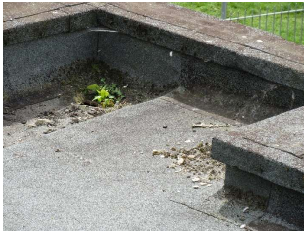
Outlet over large Vestry - Plants cleared at inspection
