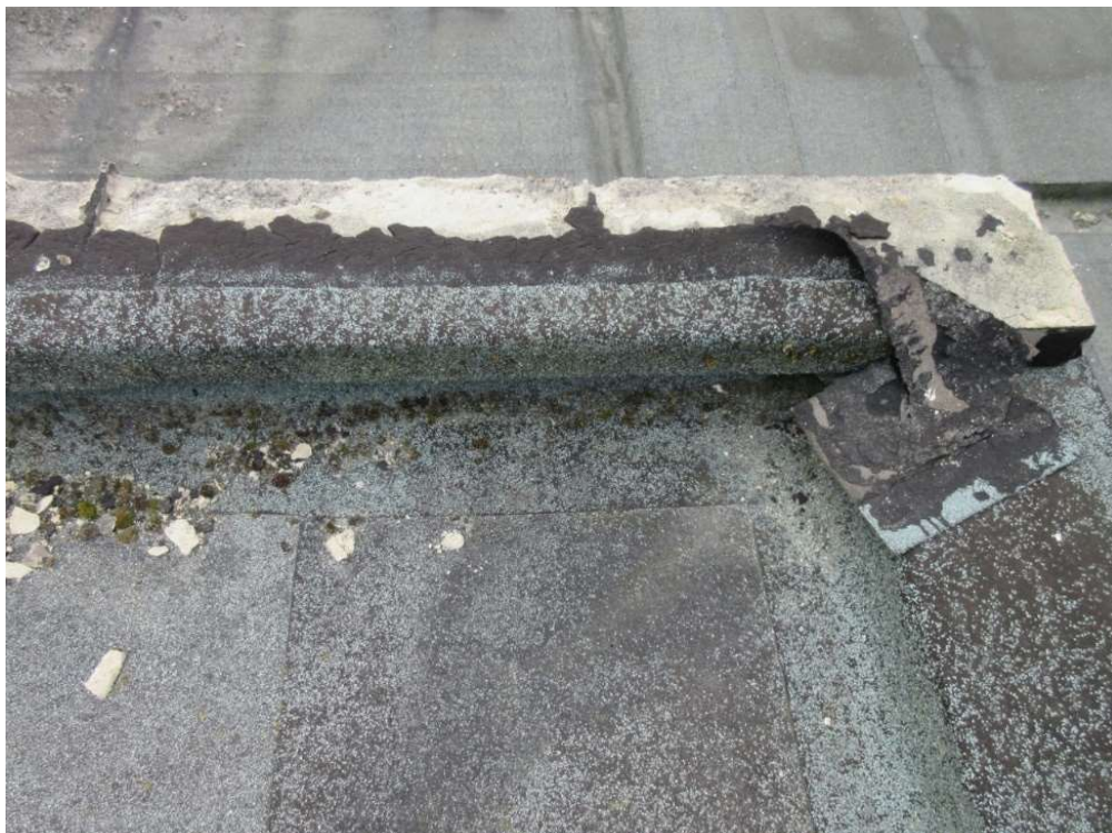
Felt peeling off top of decaying cast stone coping on end of stair roof (para 28)
