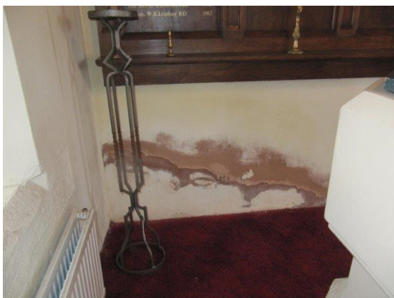
Failing plaster to West wall of Nave
