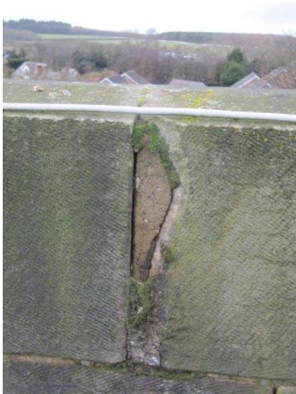
Failing mortar repair to tower parapet
