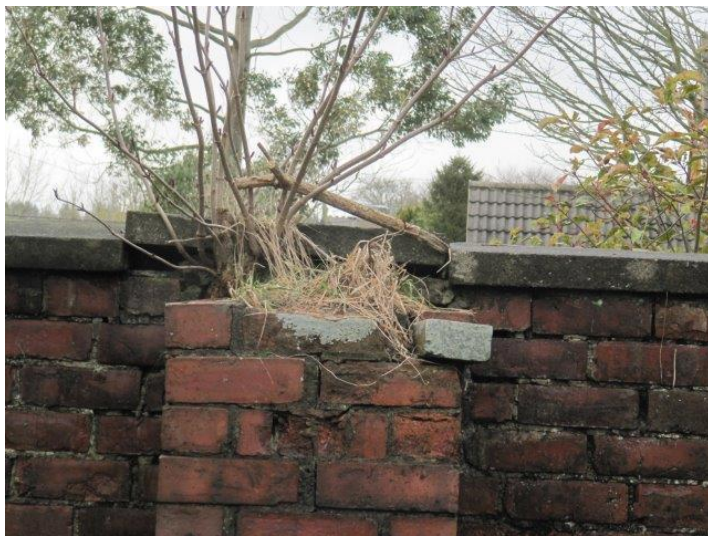
Damaged section of Western boundary with sapling, vegetation growth, open joints and lifted copings
