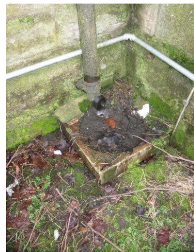
Blocked Gully to North nave
