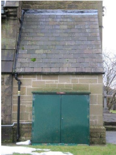
Algal growth to North WC around services cabinet
