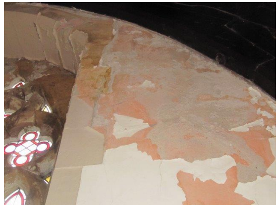
Exposed and potentially damaged plaster to East wall of Chancel
