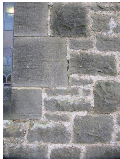
Missing mortar to North Elevation of Vestry
