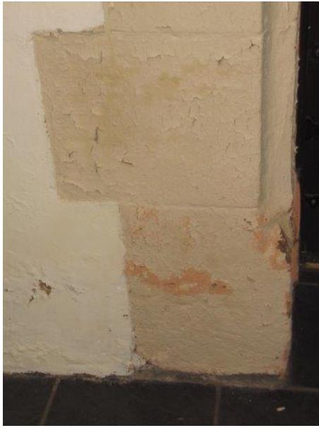
Loss of paint o porch wall and door into Nave
