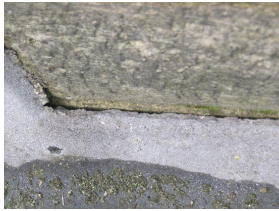
Asphalt upstand coming away from tower parapet
