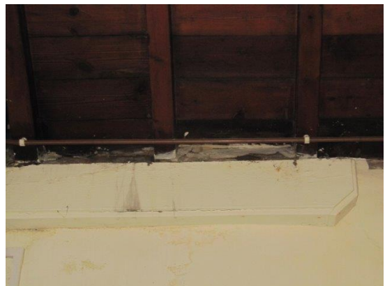
Damaged wall plate in vestry
