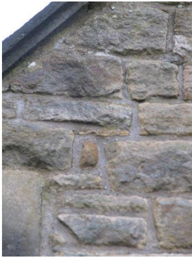
Cracking to East gable of Chancel
