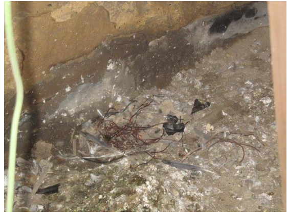
Pigeon droppings to tower
