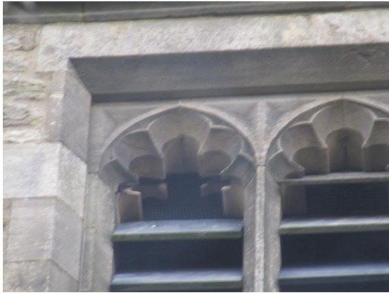
Missing louvre to South Elevation of tower
