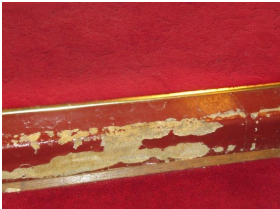
Failing paint to Chancel step revealing sanding stone behind
