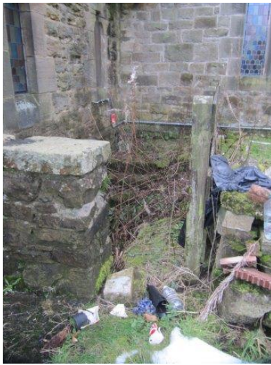
Gap in barrier to side of stairs and collection Of discarded and broken objects
