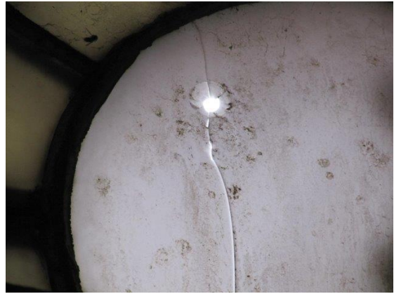
Crack and shot hole to clock face
