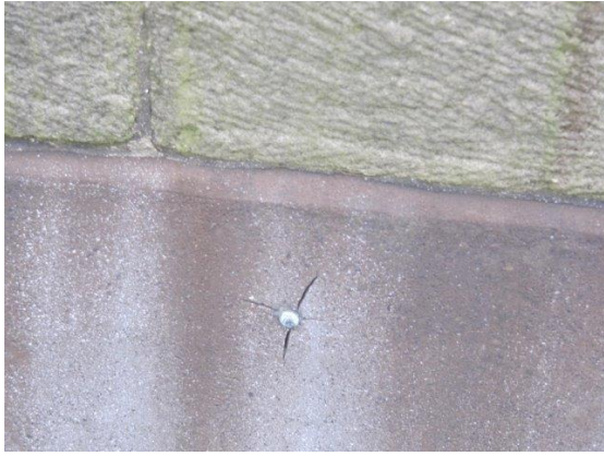
Splits in Tower asphalt around metal pin
