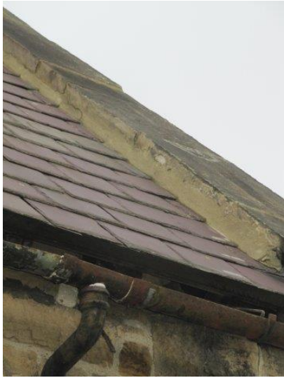
Rusting gutter and slightly sloping section of gutter to North Nave
