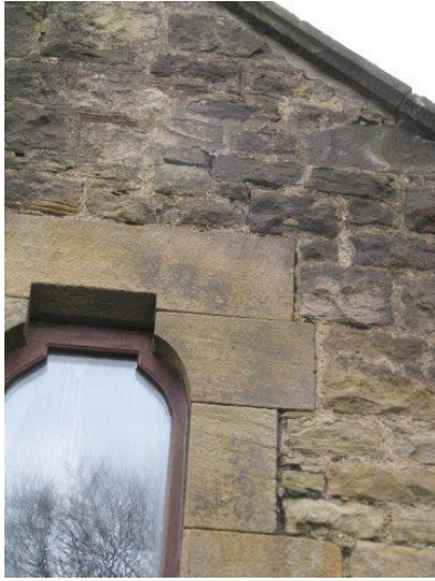
Open joints to side of North vestry window
