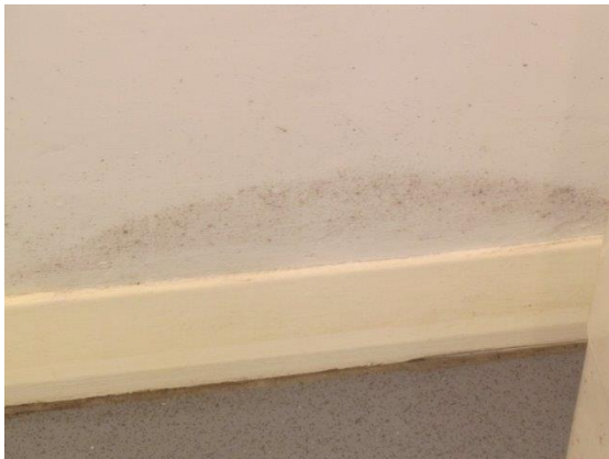
Damp/mould to base of WC wall
