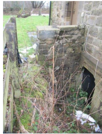
Vegetation ad debris to boiler room steps
