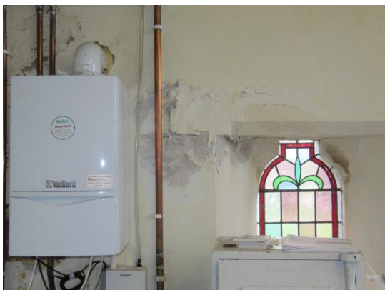
Damaged plaster behind boiler
