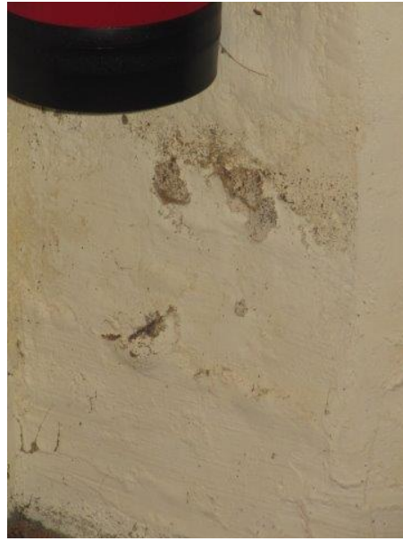
Failing plaster to base of porch wall
