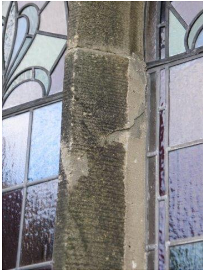
Crack to mullion North Nave window
