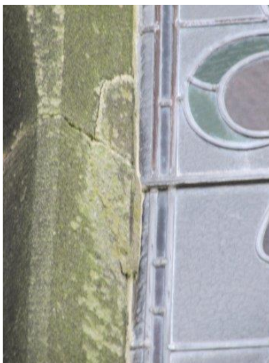
Crack to mullion East window of Chancel
