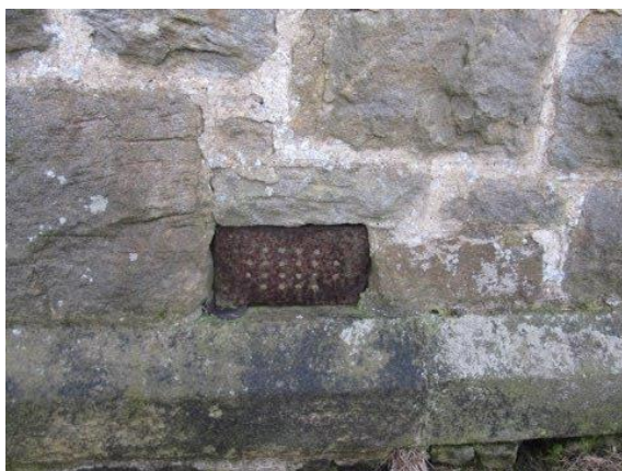
Rusting and filled vents to Vestry
