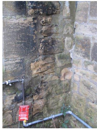
Damper wall and poor pointing to South end of West Vestry wall
