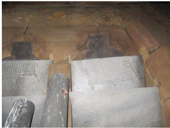
Louvred openings are only partially covered in mesh
