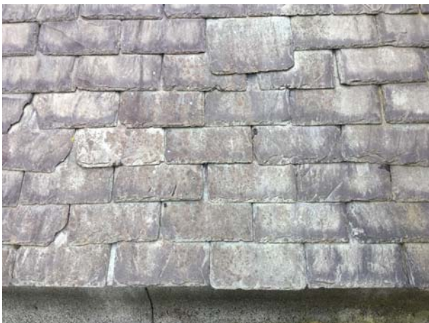
Photo 4: Slipped Nave south side
