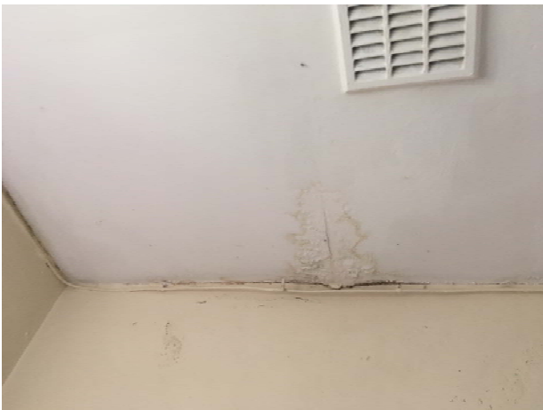
Photo 28: Water damage on Flower Room ceiling
