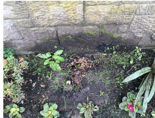
Photo 25: Leaking overflow east side
