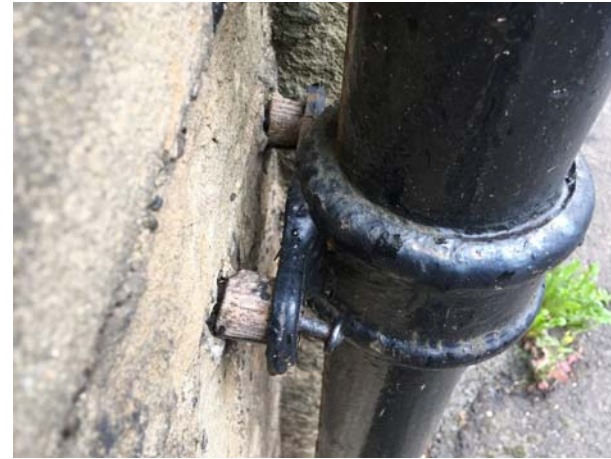
Photo 23: Loose RWP fixings
