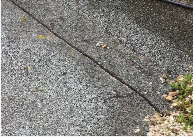
Photo 15: Cracked felt roof over Narthex
