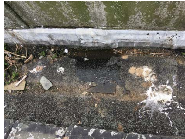
Photo 6: Spongy gutter and seagull debris on west side of North Transept
