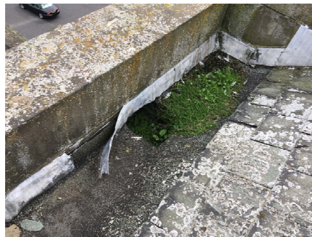
Photo 7: Blocked outlet and loose flashing on east side of South Transept
