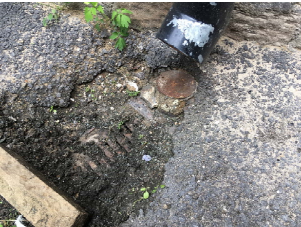
Photo 16: Blocked gully north side of Nave
