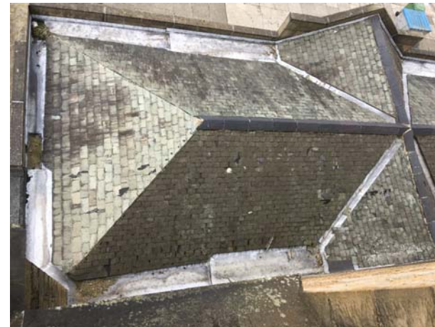
Photo 12: Many slipped, missing and broken slates over Narthex
