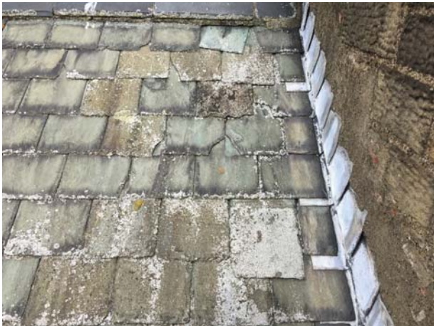
Photo 3: Slipped and broken slates south side of Nave at Transept abutment
