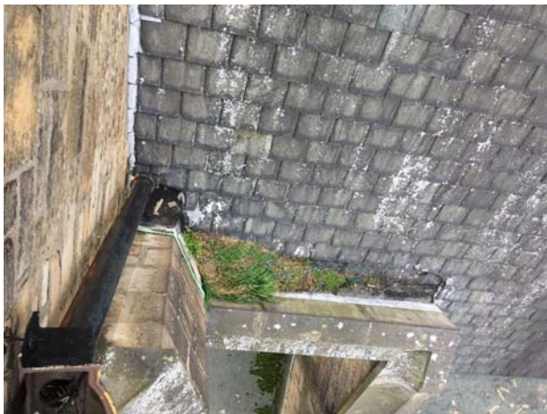
Photo 9: Debris and vegetation on north side of Nave
