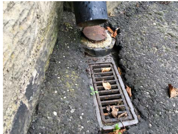
Photo 19: Discharge on south side runs to ground between macadam and gully
