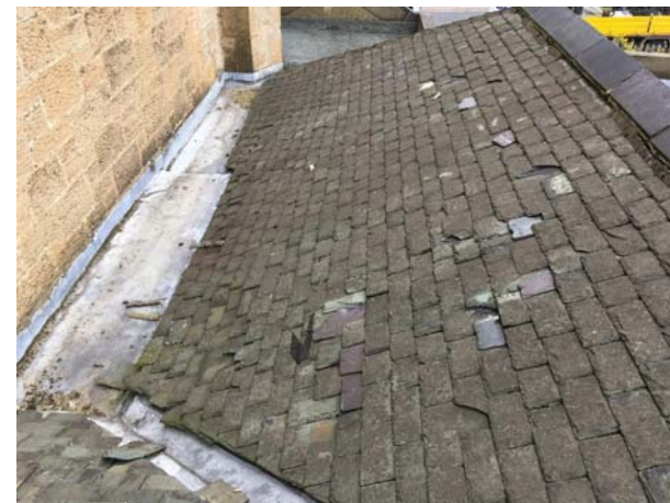
Photo13: Slipped and broken slates on east side of Narthex
