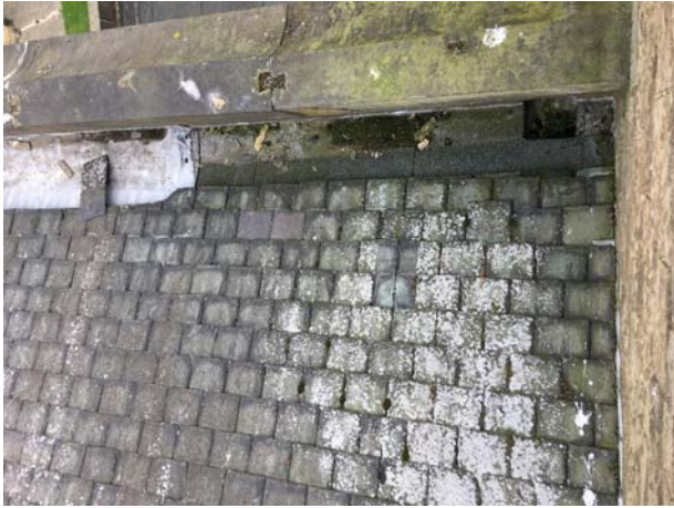
Photo 2: Slipped slate over organ
