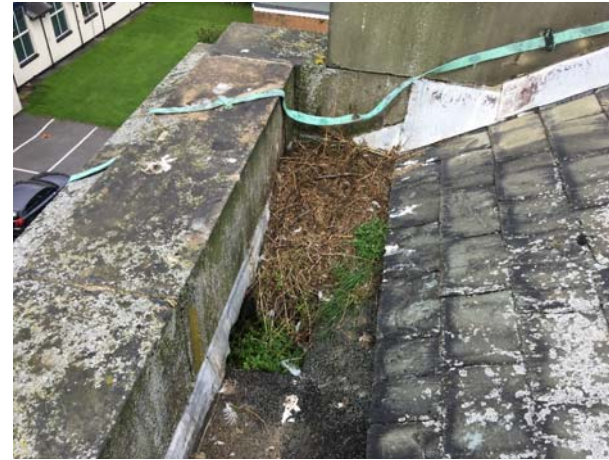
Photo 5: Seagull debris has blocked outlet on west side of North Transept
