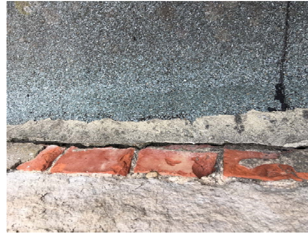
Photo 11: Absent flashing on southwest corner of South Transept allows water to run down behind felt roof
