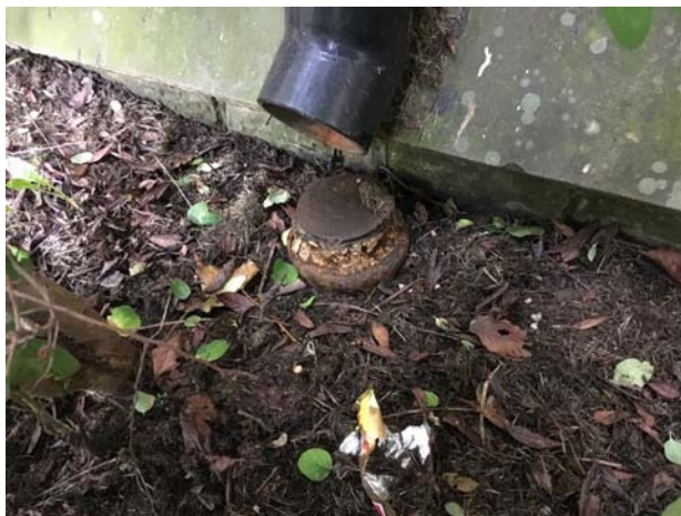
Photo 22: Blocked gully behind bush on south side of Nave
