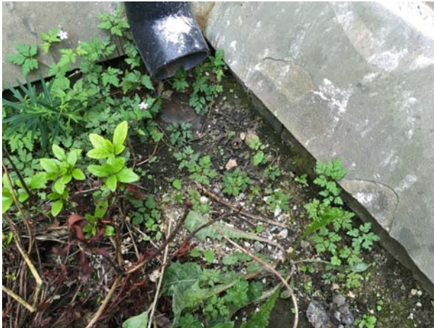
Photo 21: Blocked gully on south side of Nave
