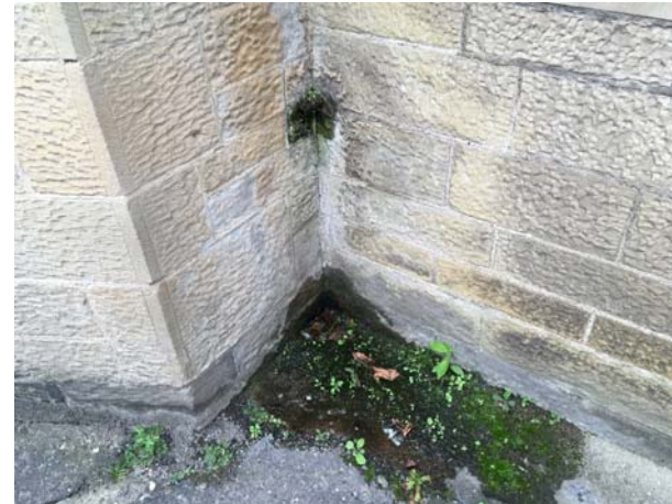
Photo 24: Leaking overflow south side
