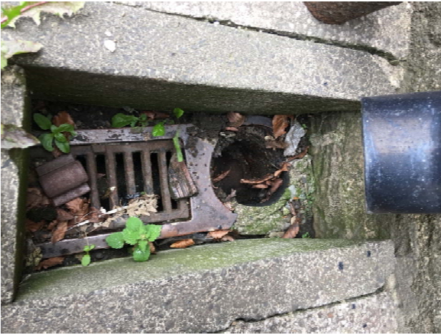
Photo 20: Discharge on south side runs to ground between concrete and gully
