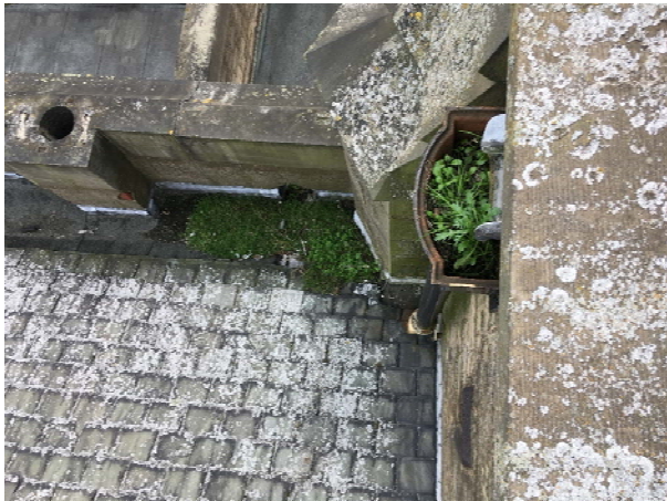
Photo 8: Blocked hopper head and outlet on east side of Chancel
