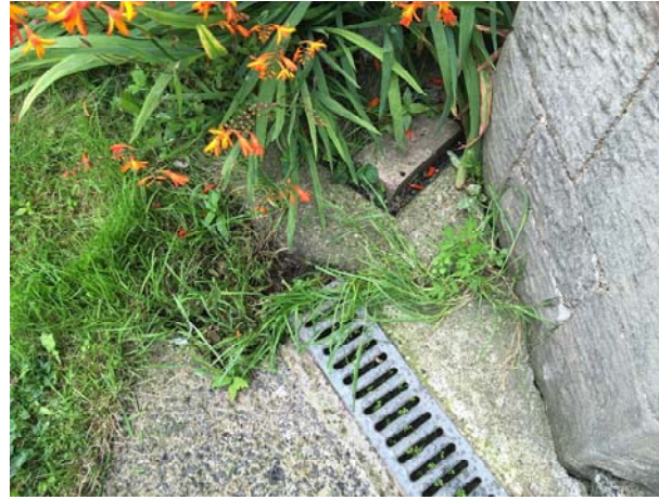
Photo 17: Blocked gully north side of Undercroft
