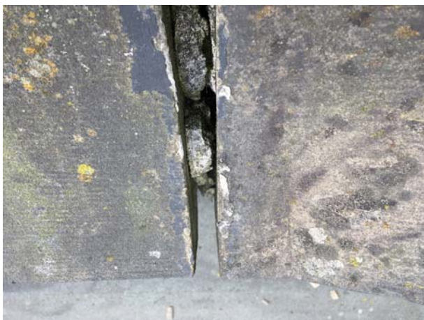
Photo 10: Open joints between wall head copings
