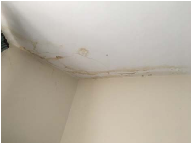
Photo 27: Water damage on Vestry ceiling
