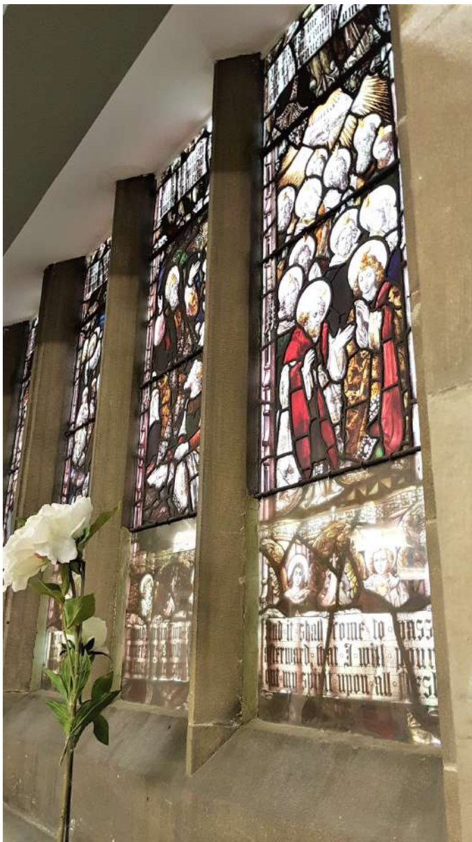
Re-pointing and minor repairs to glazing required to west window
