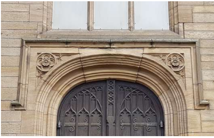
Key stone dropped over main west doorway - not progressed
