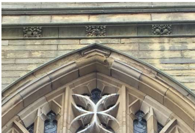
Weathering of masonry below open-jointed or inadequate stringcourses and to bottom roll of hoodmoulds where water is penetrating. Ideally all strings and hoodmoulds should be capped with lead
