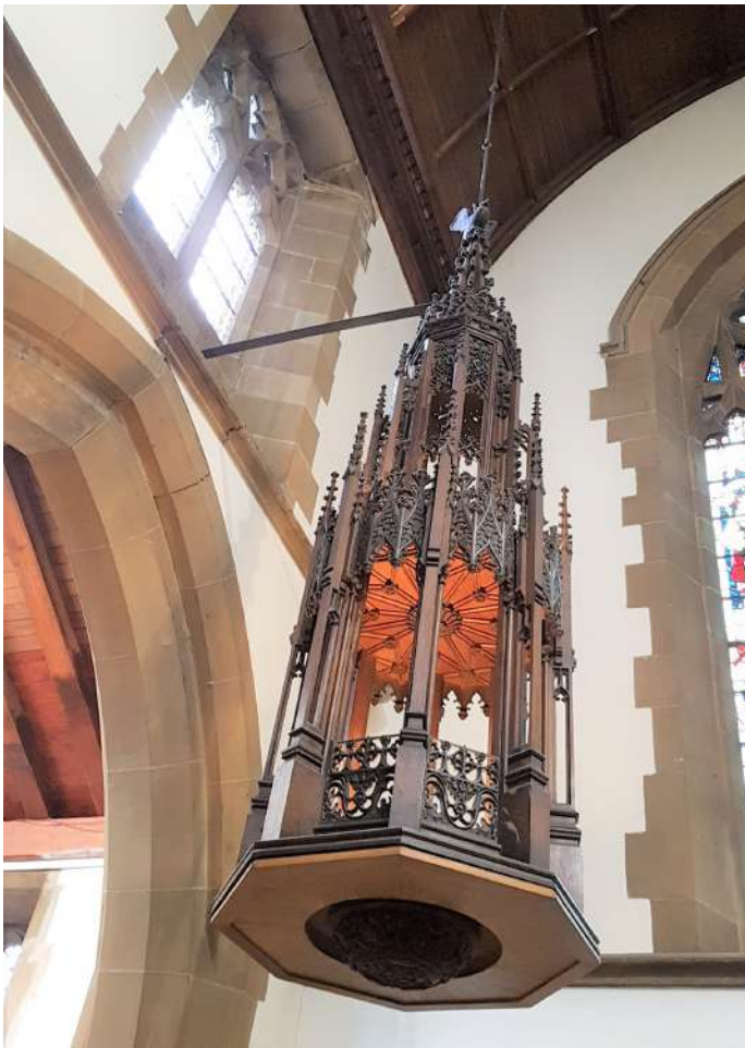
Dry-rot found and timber / gutter over repaired. Iron bracket holding the font cover has cracked the masonry at the window cill - monitor
