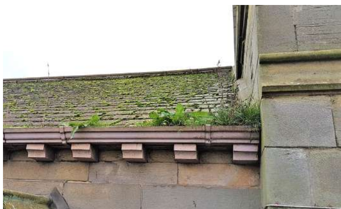
Vegetation in Chancel eaves gutter
