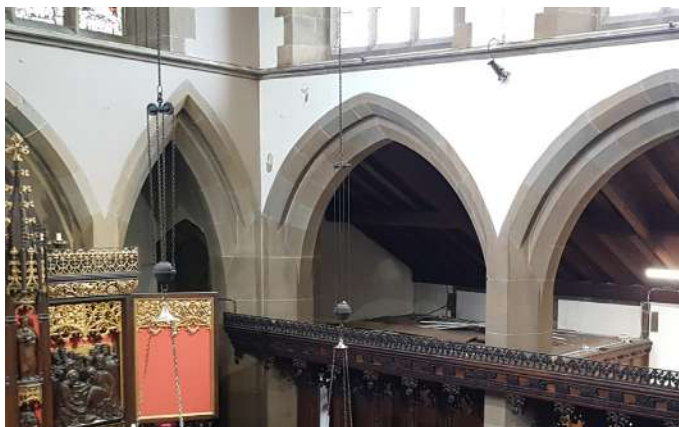
Peeling paintwork indicating damp in south-east corner of chancel (coincides with missing flashings externally)
