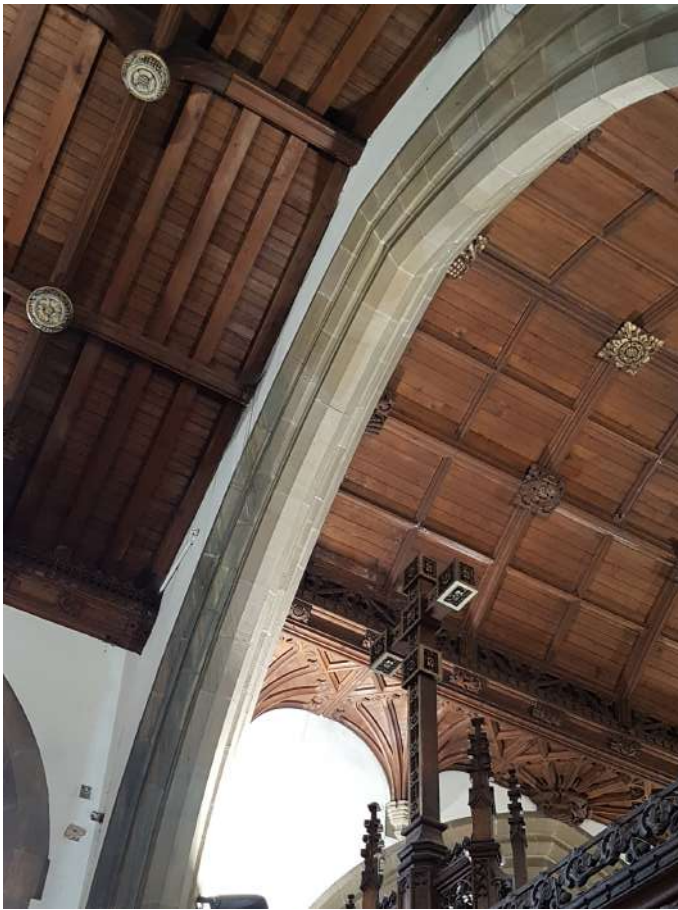
Leaks over chancel arch/crossing arches, staining from purlins - monitor
