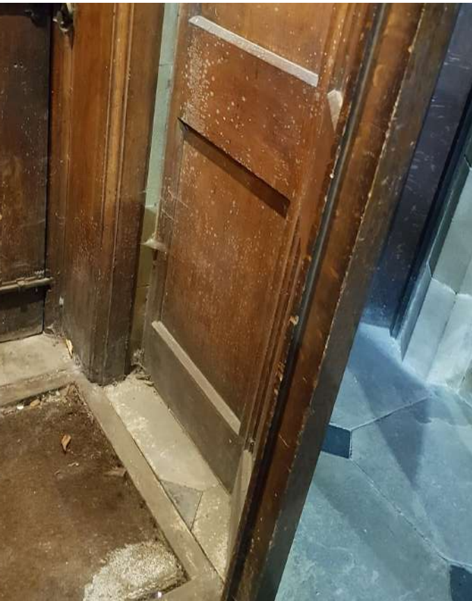
Mould to inside of north aisle draught porch, on both timber and mat
