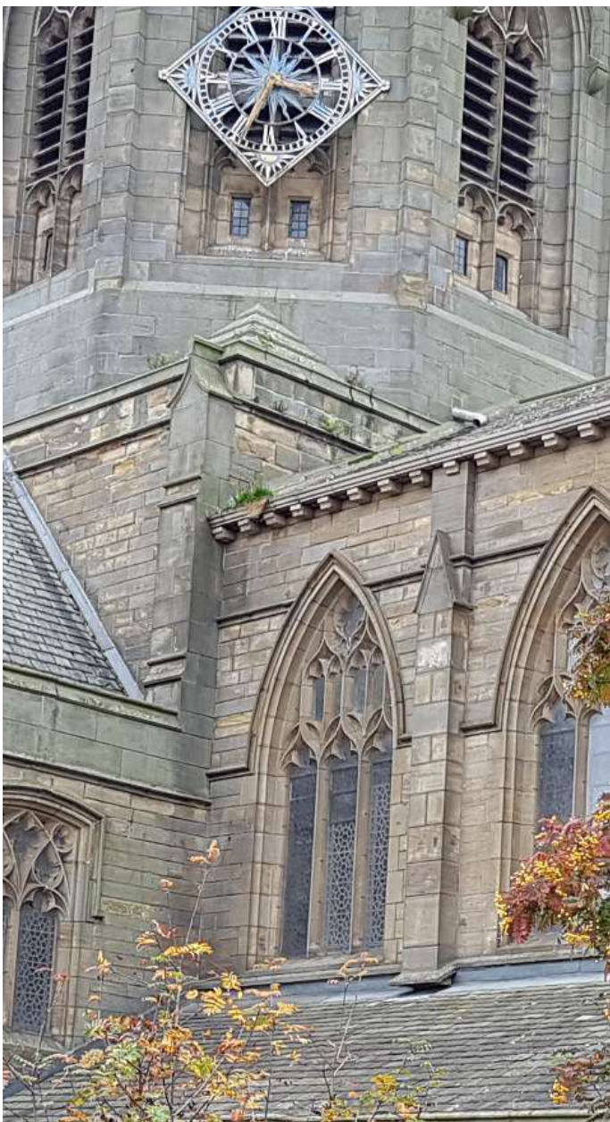
Vegetation in tower broaches, vegetation in high-level gutters. RWP discharging onto south chancel roof
