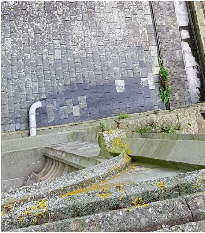
Discharge from tower onto Chancel roof - heavy vegetation directly below discharge
