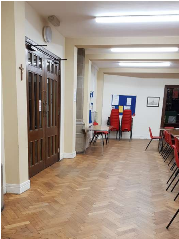
Community hall - woodblock floor required easing and re-bedding in localised areas where lifting
