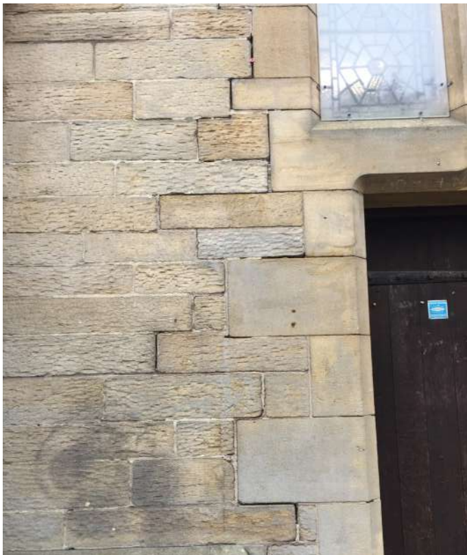
Localised cracking through joints to west of garden door
