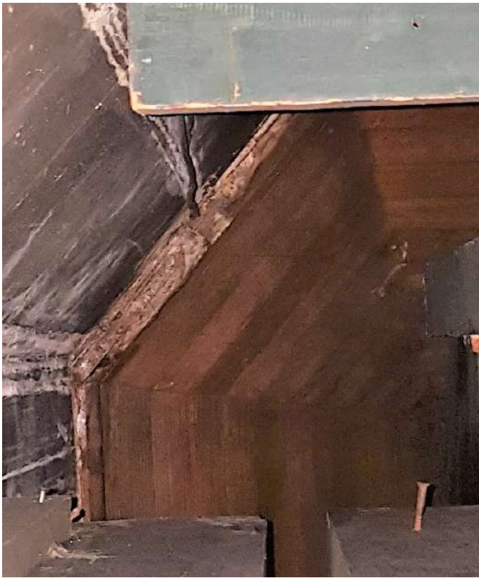
Rotten timber to underside of organ loft roof, behind organ pipes (looking up)
