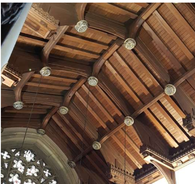
Lighting vastly improved since last inspection - new lighting installed
