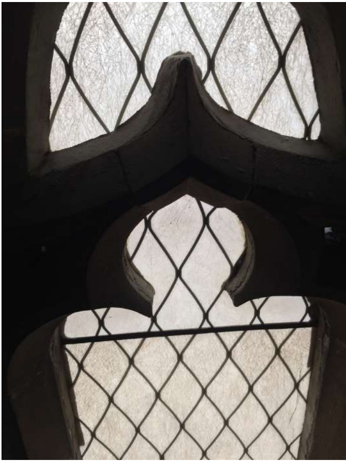
Fibreglass glazing in office - thermally very poor, room very cold and barely usable
