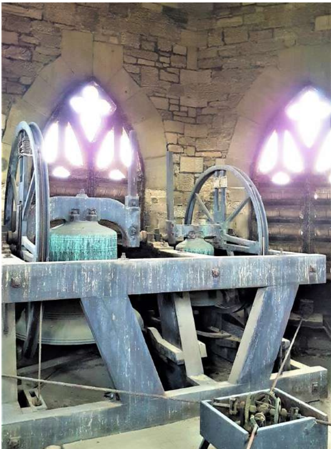
Timber bell frame on concrete floor - good condition though would benefit from a clean
