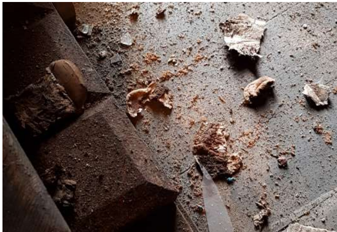
Remnants of large fungus, fallen from underside of organ loft roof (noted in last QI, located on timber soffit boarding)
