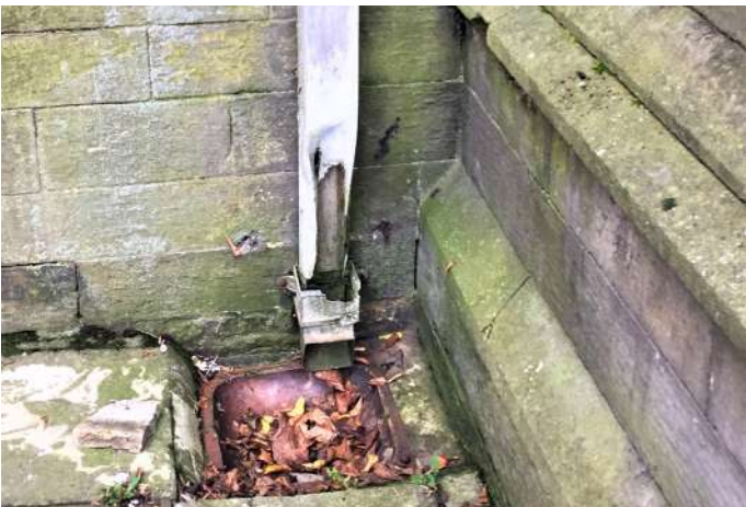
Damaged lead downpipe discharging into gully
