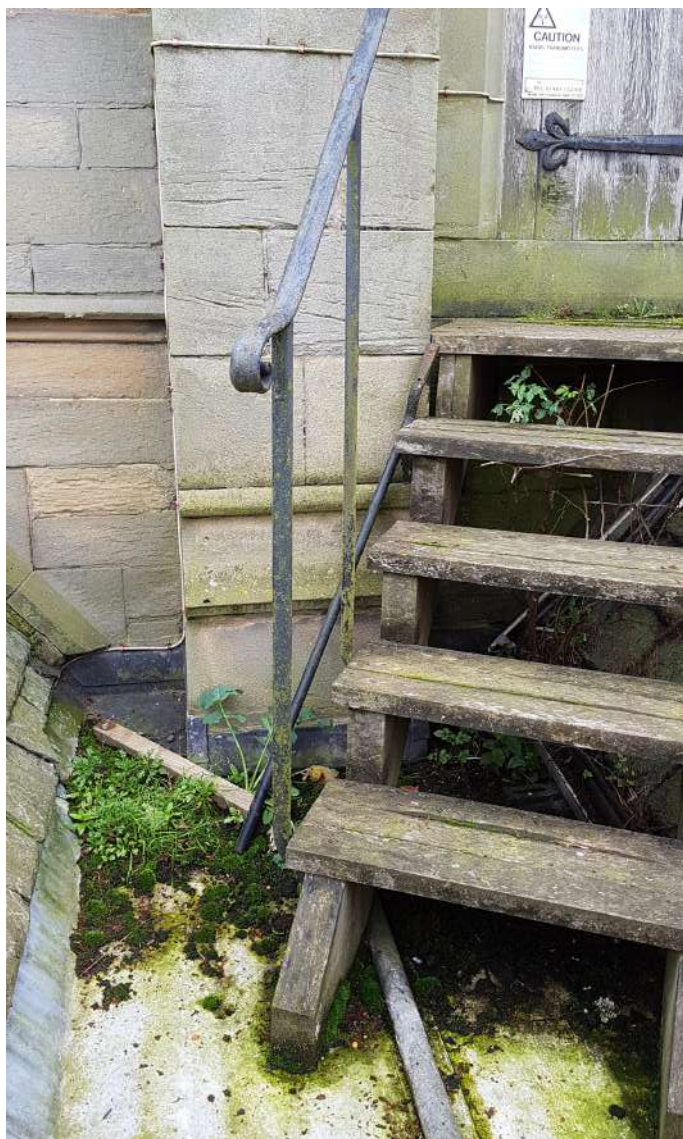
Lead roof between organ loft and north transept at end of life. Steps unsteady. Vegetation build up.
