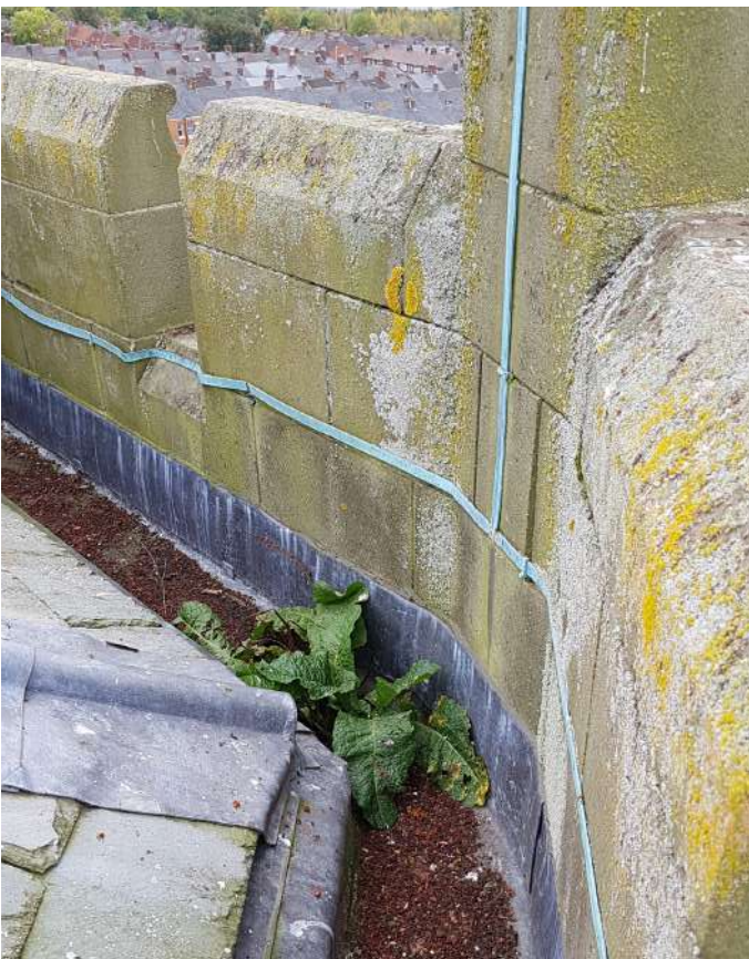
Tower - gutters full and outlets blocked with vegetation
