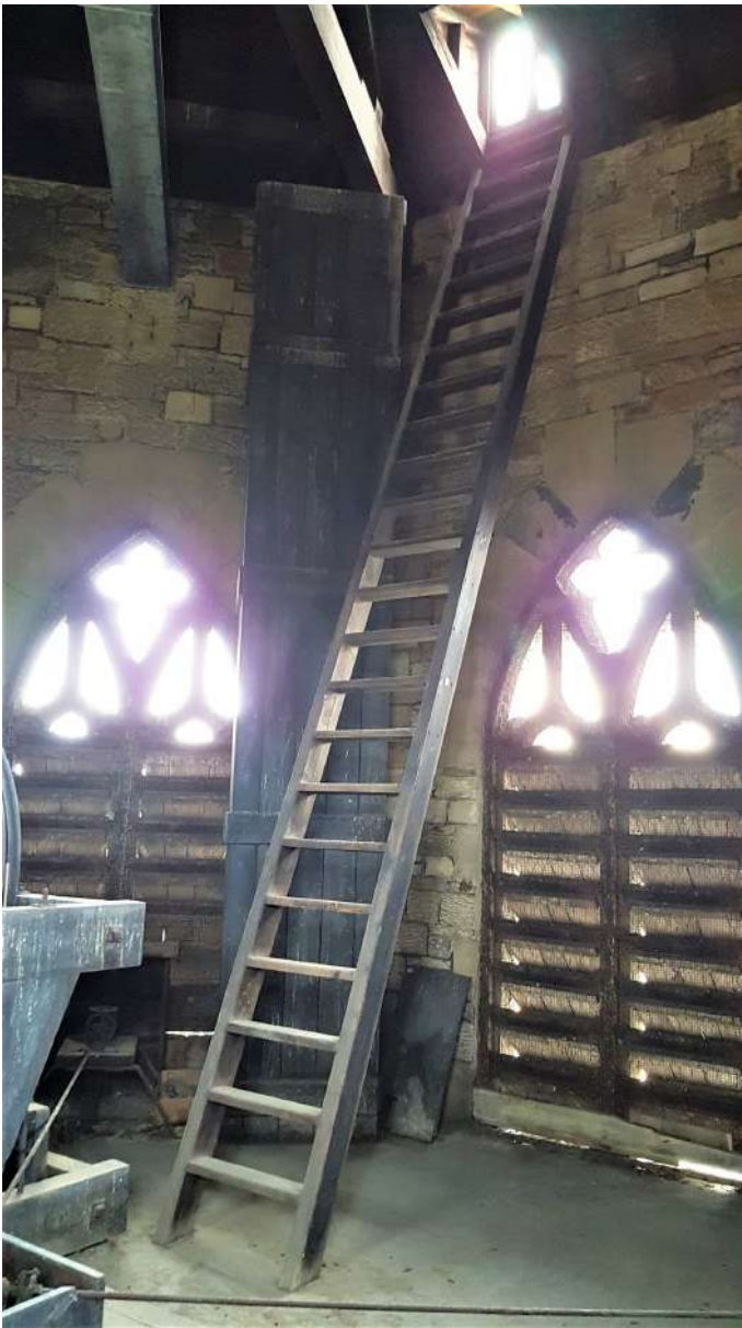
Access to tower roof. Add sign to warn users about the exit onto the parapet so they understand the risks
