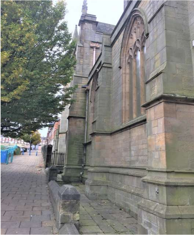
Railings missing from western end of north boundary wall. Areas behind boundary walls kept clean and tidy
