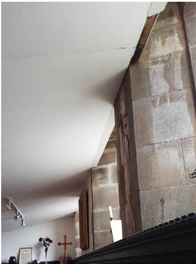
Choir vestry - damp to windows and staining from water ingress above - false ceiling and wall panelling hides issues
