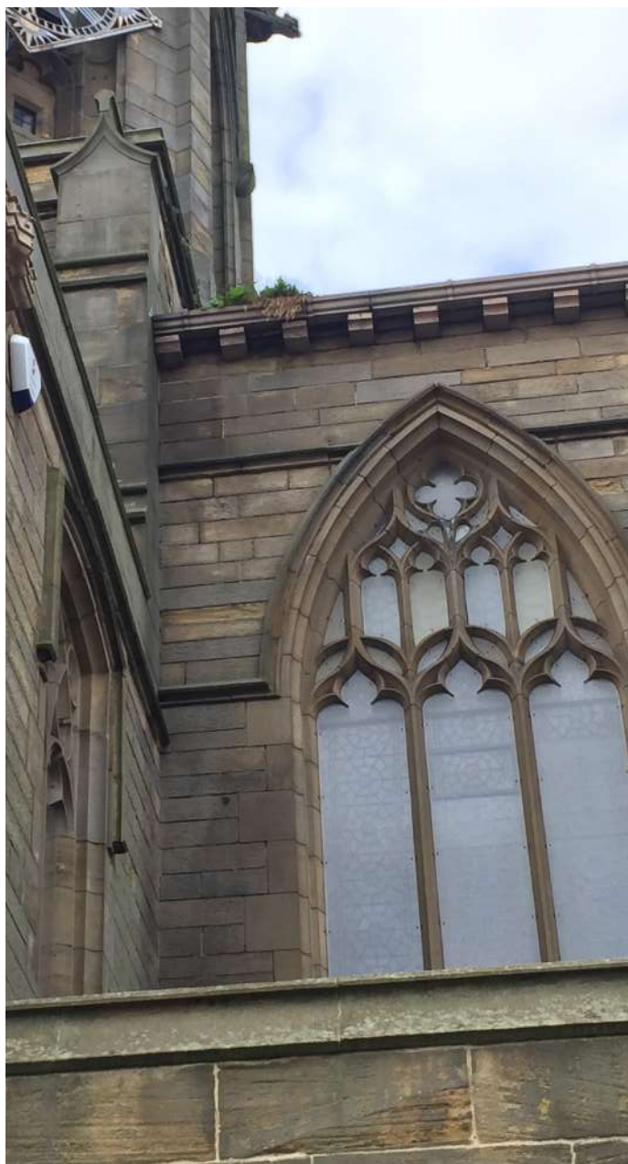
Polycarbonate sheets on exterior of windows - well fitted and neatly cut, though now clouding and would benefit from renewal in the long-term
