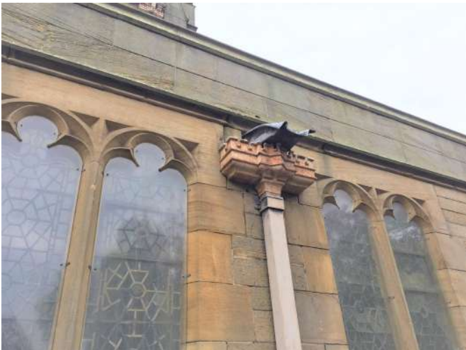
Rusting hoppers and disfigured lead chutes from thieves trying to remove/pull out
