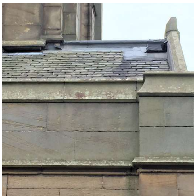
Two areas on south chancel roof where flashings have been peeled back by thieves looking for lead
