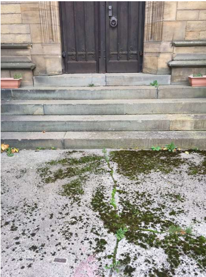
Cracked concrete to front of west door would benefit from repair and steps re-pointed to resist weed growth in gaps
