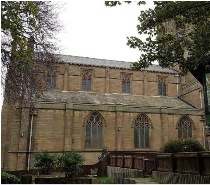
South aisle in poor condition
