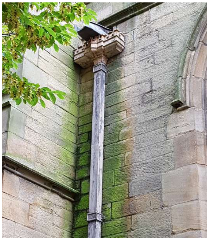
Rainwater spilling down masonry
