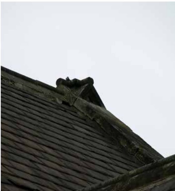
Misaligned copings to east end of Nave
