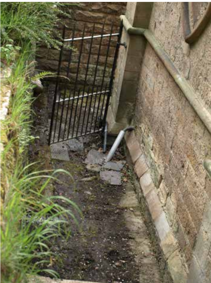
Gully at south west corner, collecting water from roofs, kitchen sink and bank. Surface water drainage in this area is poor.
