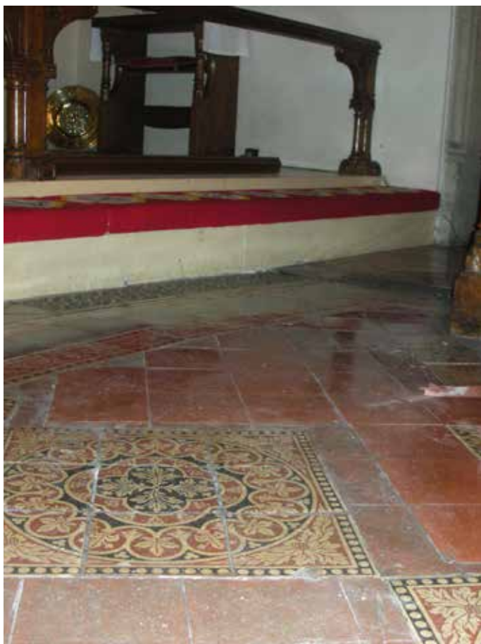
Tiles to quire and sanctuary
