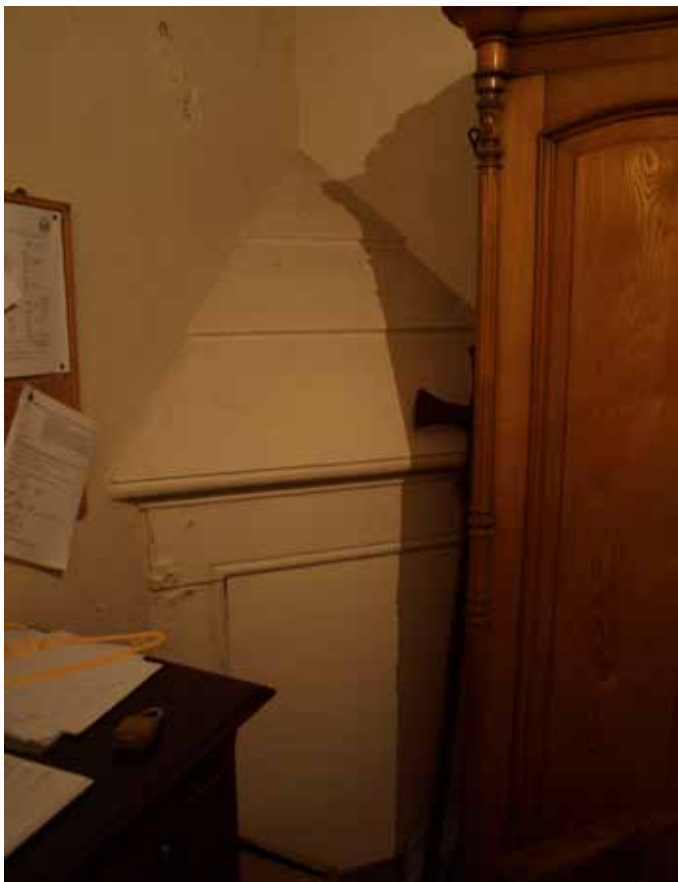
Ventilation of the Vestry chimney should be considered
