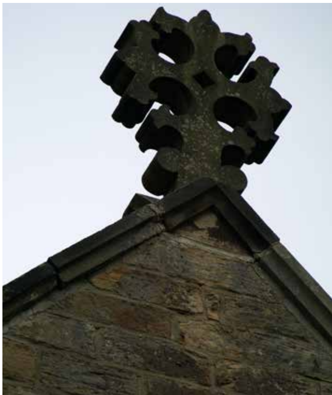
West end cross finial has been re-bedded, but the mortar is cracking away in the joints again. Other open joints in coping.
