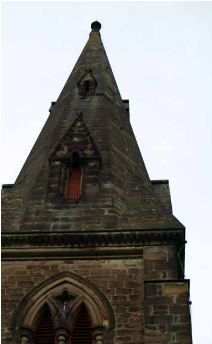
Tower masonry generally appears in good condition when inspected from ground level
