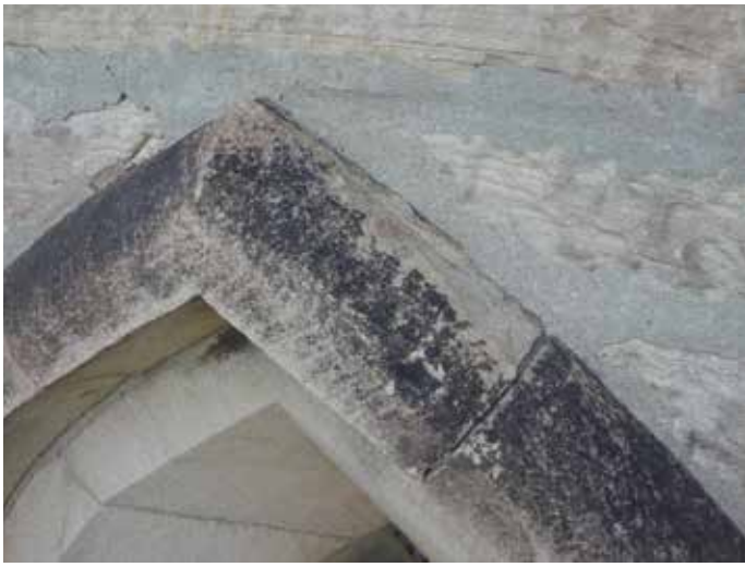
Spalling stonework on top of hood-moulding, cementitious pointing to the walling masonry adjacent
