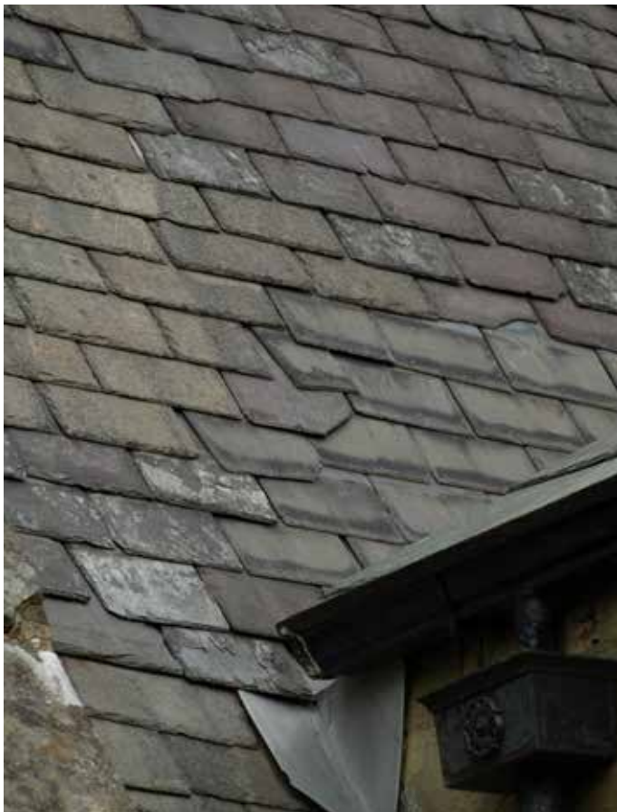
Displaced slates on Vestry roof - an inadequate repair
