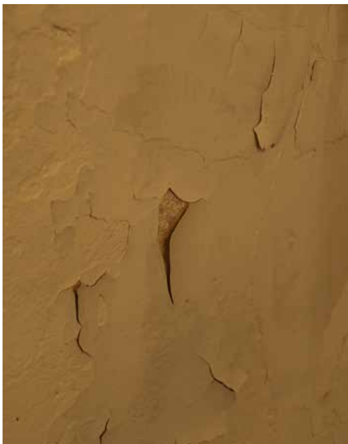
Peeling paintwork is widespread
