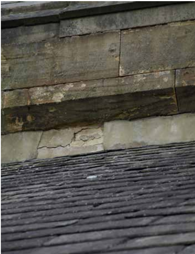
Parapet gutter of north pitch of nave, with cement mortar fillet/ render, now deteriorating
