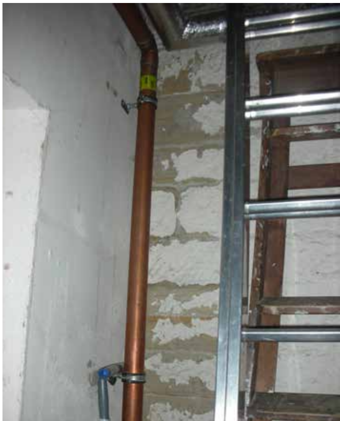
Paint directly onto stonework in choir vestry is peeling. This should be allowed to fall away and not over-painted.
