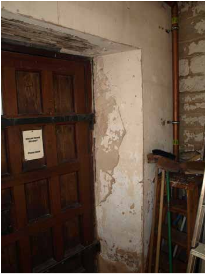
Failure of plasterwork around external door to choir vestry
