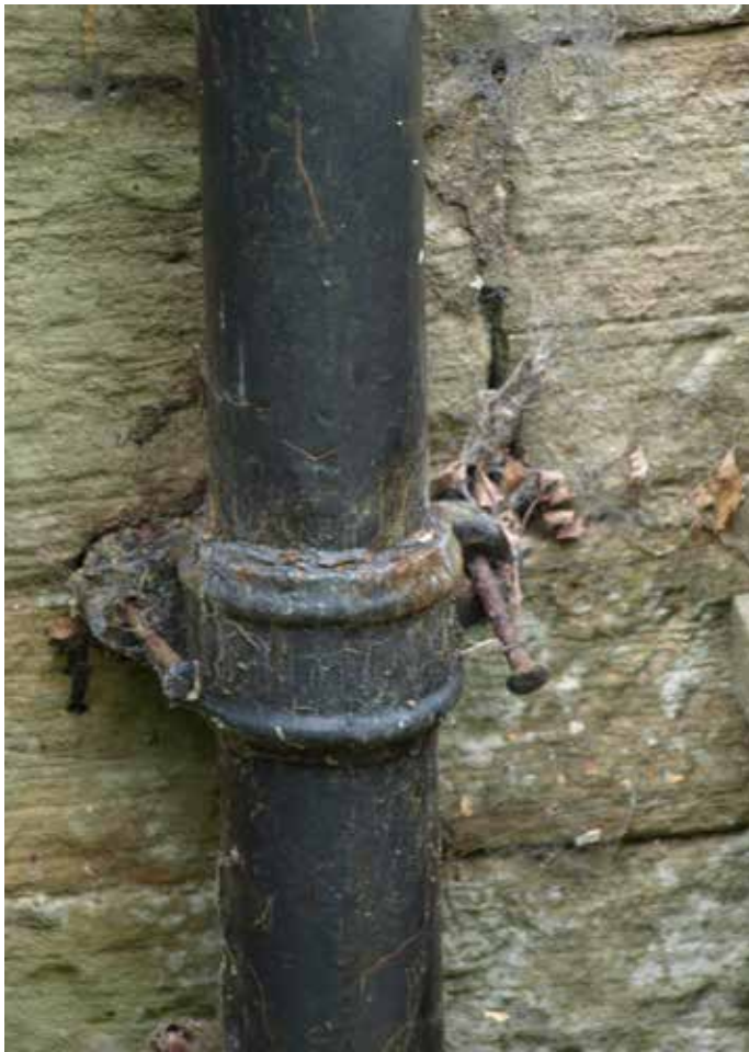
Some rainwater goods need re-fixing and re-painting
