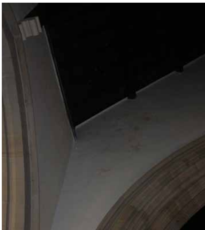
Damp staining over chancel arch, from nave
