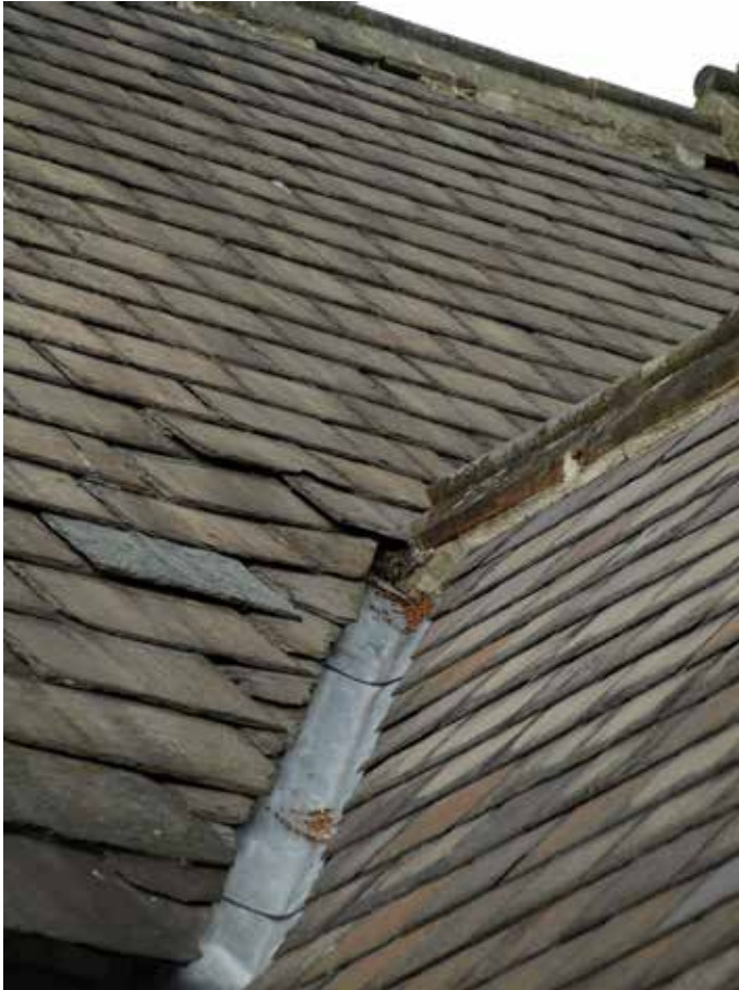
Dislodged slates at abutment of south transept
