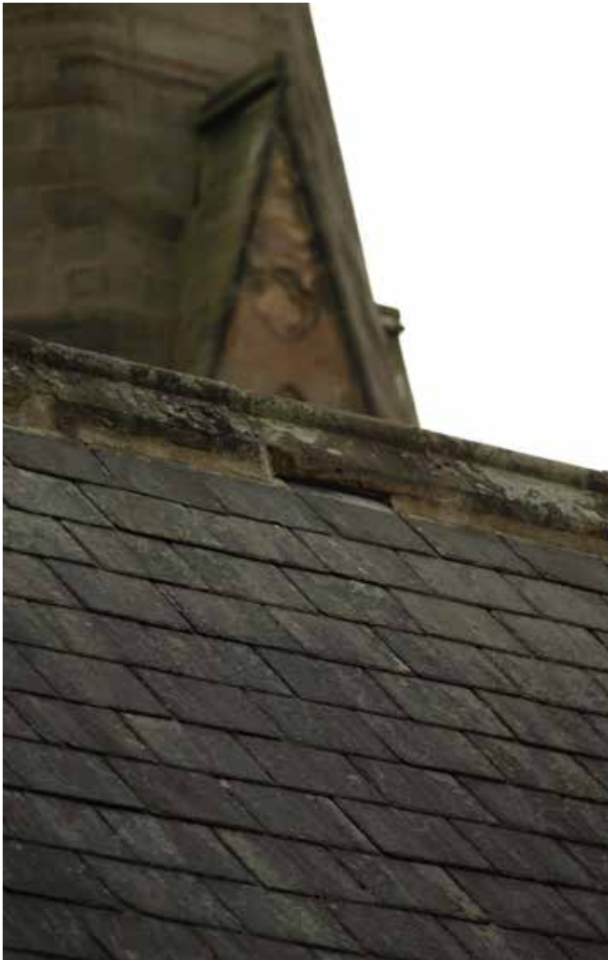
Lost pointing to south transept ridge
