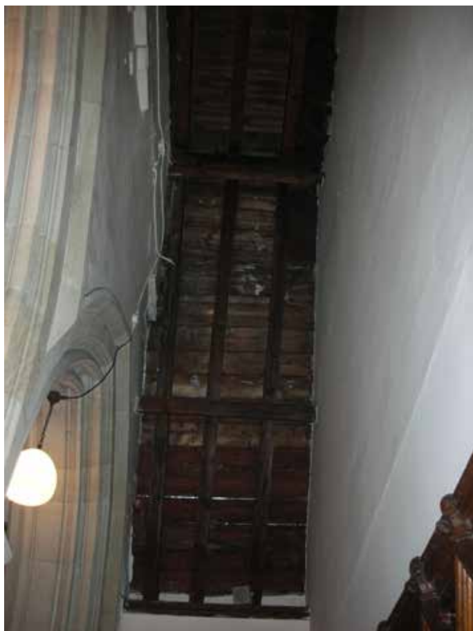
Roof over north stalls - lead theft caused major water ingress, now repaired
