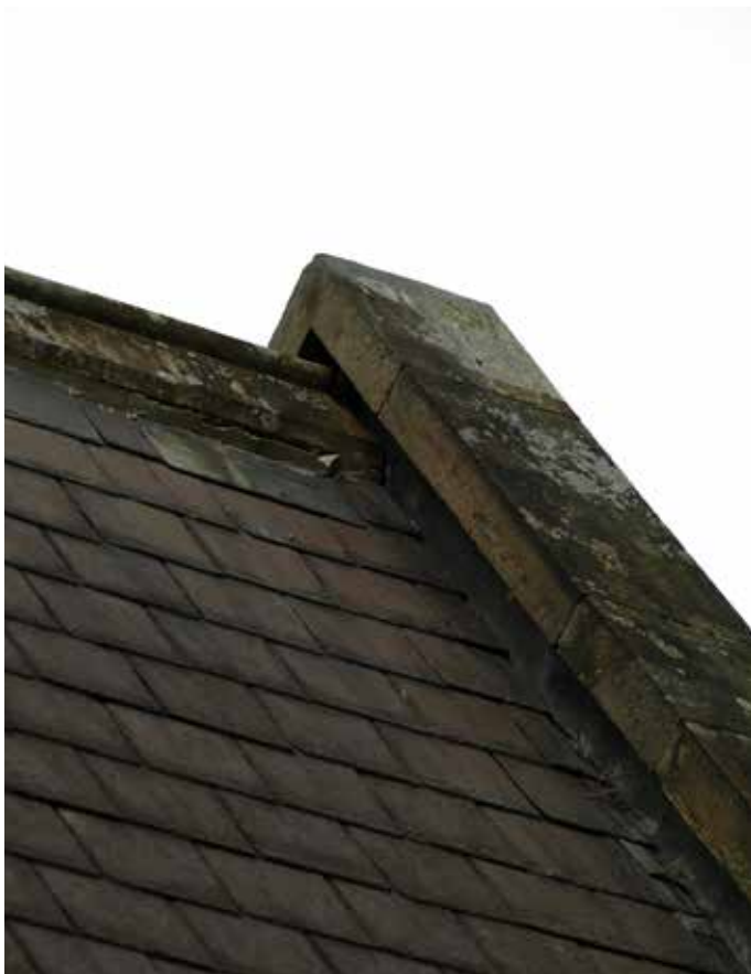
Displaced ridge pointing to Organ Loft
