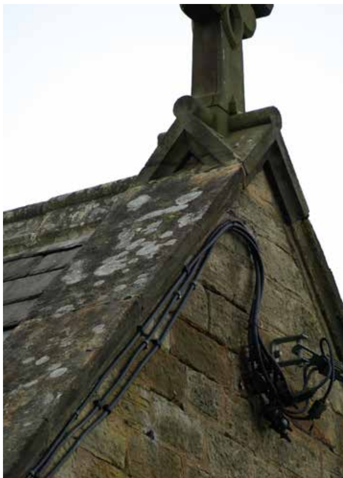
Split shaft to cross finial, and open joints in wall masonry
