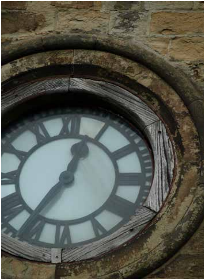
Glazing to clock face displaced, surround deteriorating
