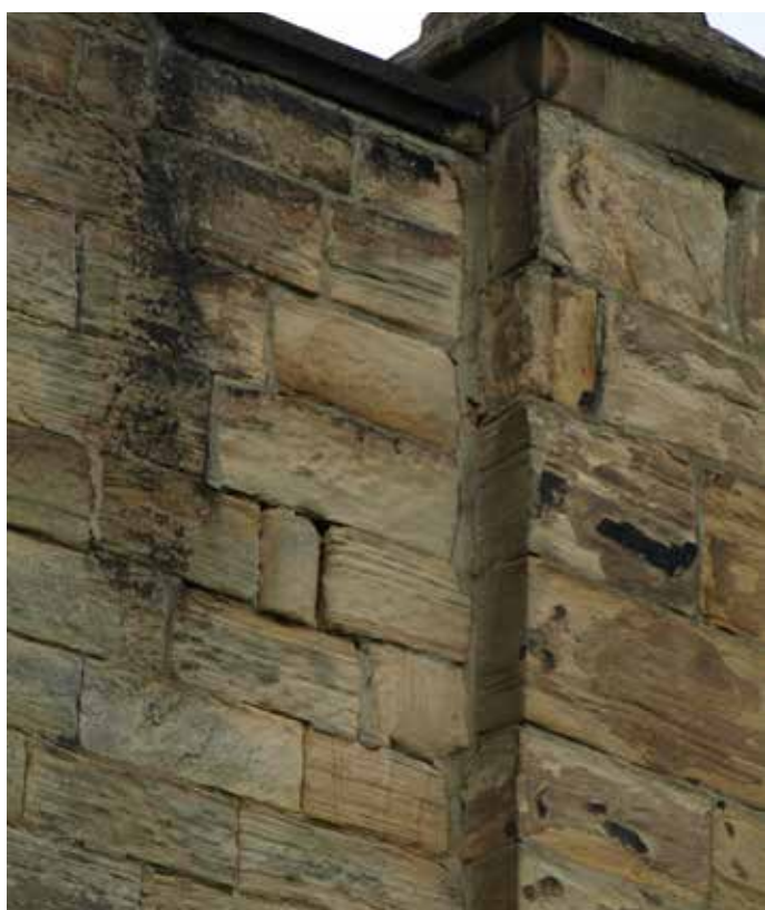
Open joints in vicinity of redundant chimney to west gable
