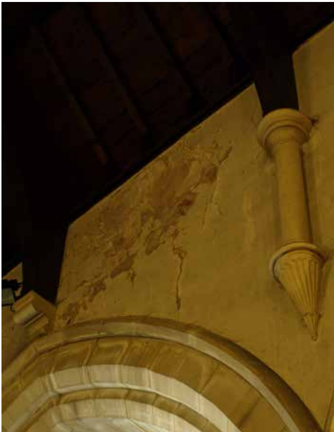
Damp staining to Nave walls at high level
