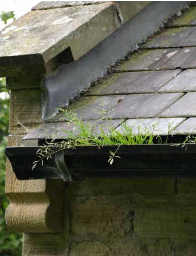
Gutters require frequent cleaning to prevent vegetation taking hold
