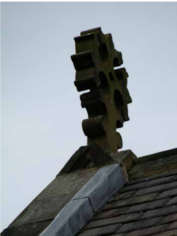
Mortar fillet to top of coping flashing cracked - a poor detail
