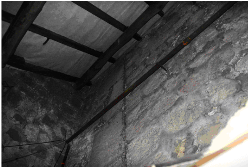
Roof space above the Vestry, looking north-east, showing the south-western angle quoin of the Saxon nave.
