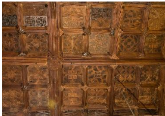
Panels in ceiling
