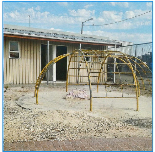
Work pending: Redundant climbing frame to be removed and ground area to be levelled and artificial grass laid.
