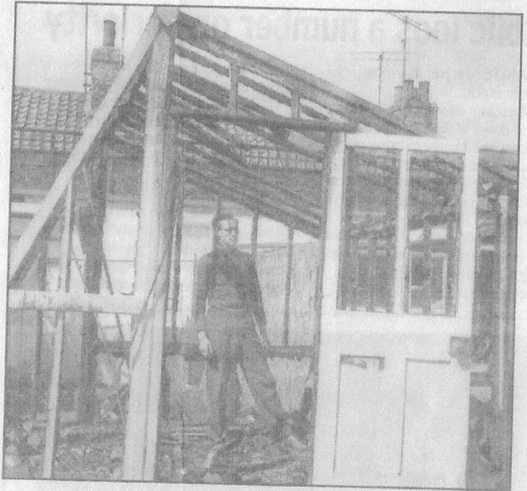
Robert Tidswell inspects the damage at his shed in Gosberton.
