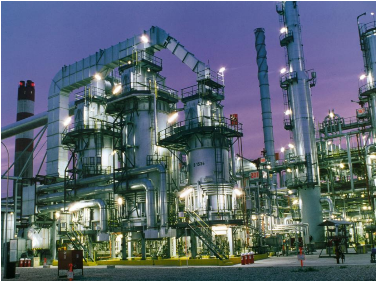
Oil Refinery Plant
