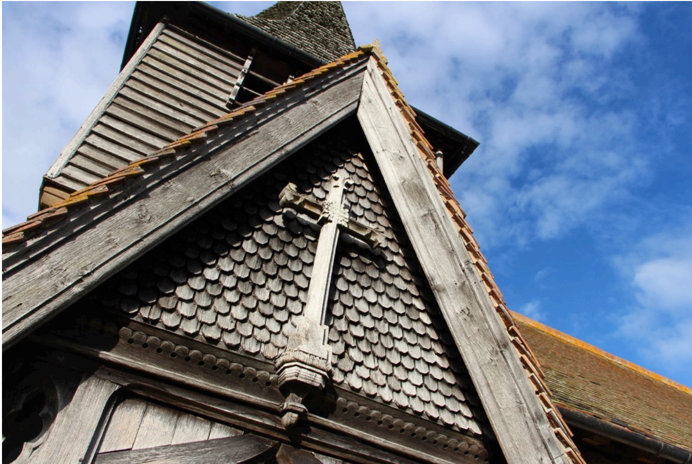
One of the highlights of St John the Baptist, Boraston, is the wooden 'scaling' on the porch.
