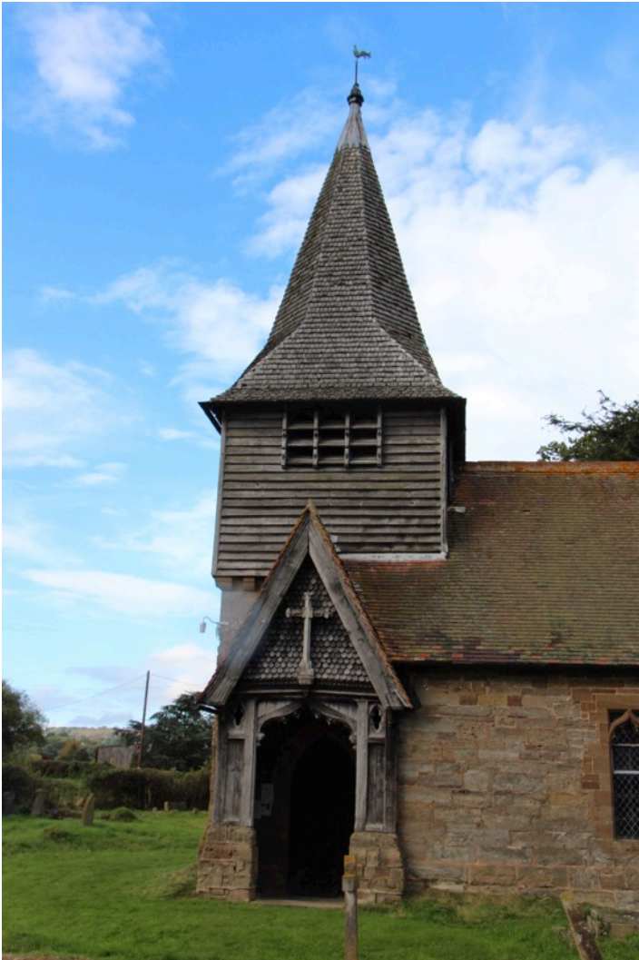
The tower at St John the Baptist, Boraston, clad with wooden slats.
