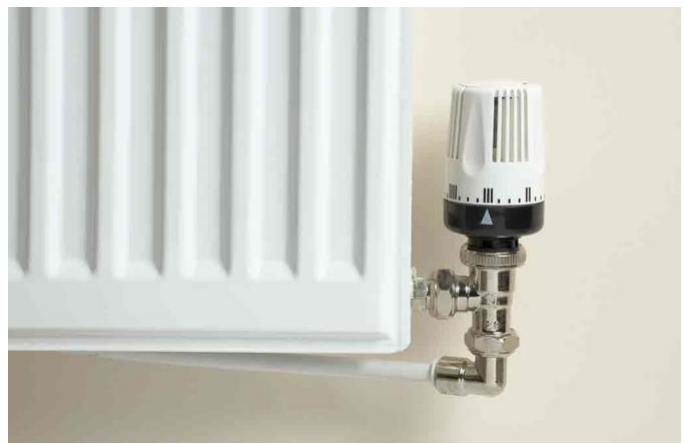
Figure 4 - Example of a TRV in situ
