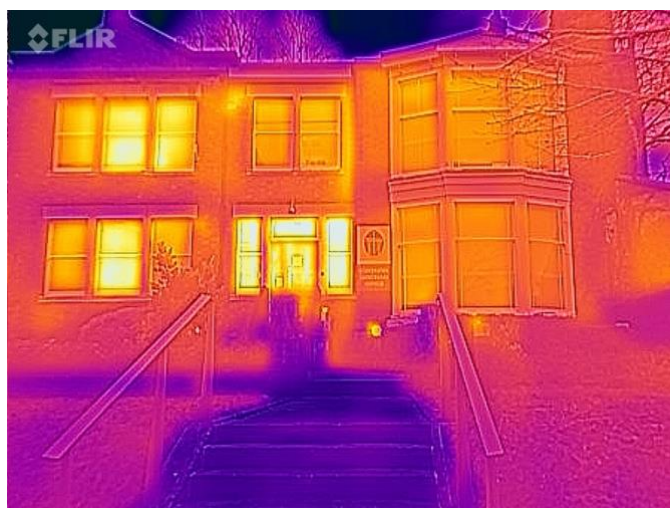
Figure 13 – Thermal radiation image of the Diocesan Offices
