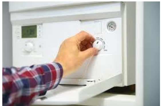
Figure 2 – image of a boiler
