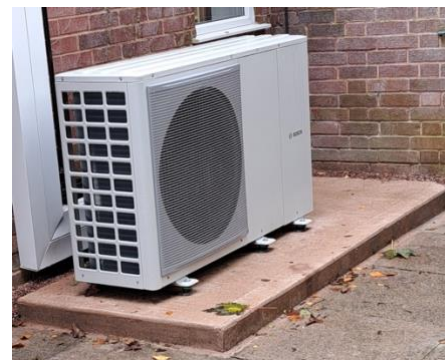
Figure 9 – An air-source heat pump in-situ at a Vicarage in our Diocese.
