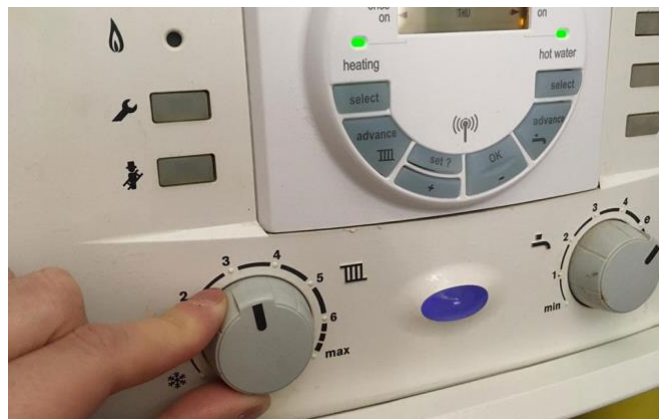
Figure 3 - Example of a person adjusting the boiler flow temperature
