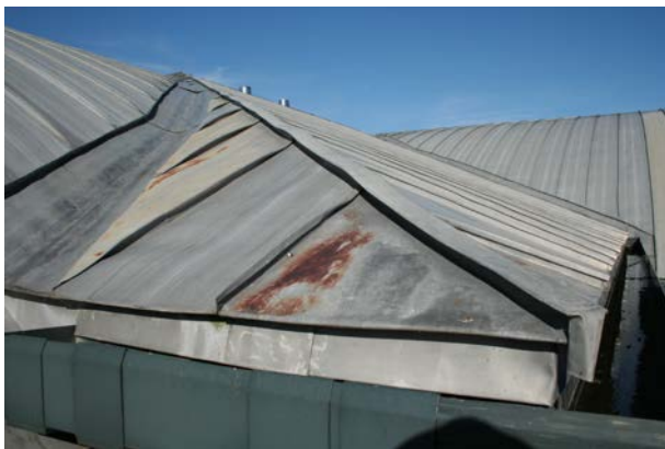
Discolouration of lead rich terne coated stainless steel
