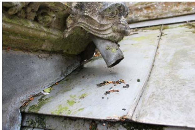
Awkward detail at verge with water running into upstand
