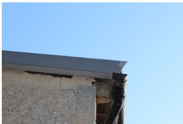
End of fascia with acute corner and incomplete closure
