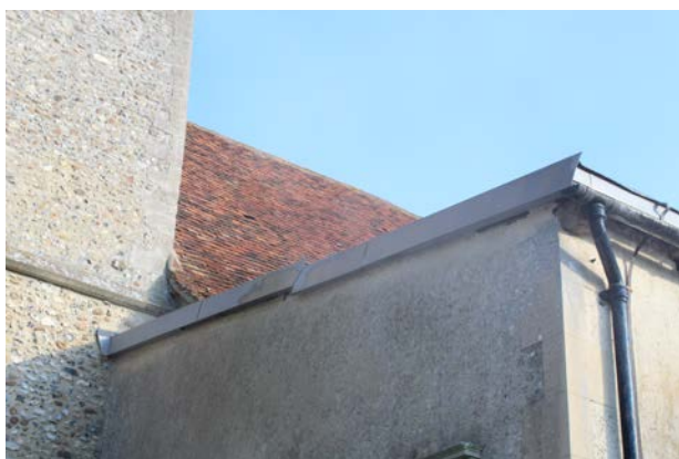
Straight verge fascia contrasts with uneven masonry
