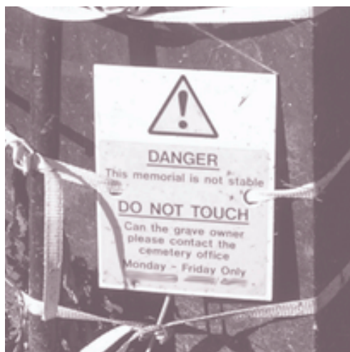
Notice on unsafe memorial
