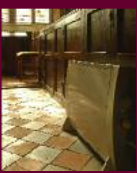
If portable heaters are required they should be of the convector or fan assisted type with a thermostatic cut out.
