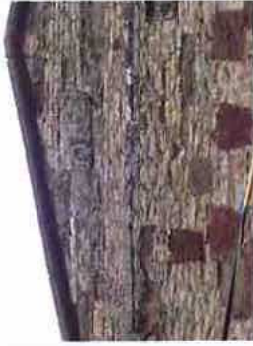
Deep point masonry bee holes in stonework.
