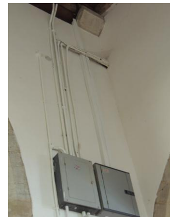
The location of electrical equipment and wiring runs all needs careful consideration with professional advice
