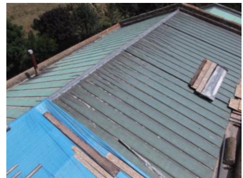
Copper Roof part stolen The remainder of that roof has been stolen since the picture was taken.
