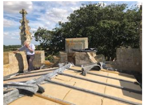
Lead Tower Roof stolen
