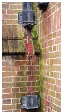
Lead Rainwater Pipe
