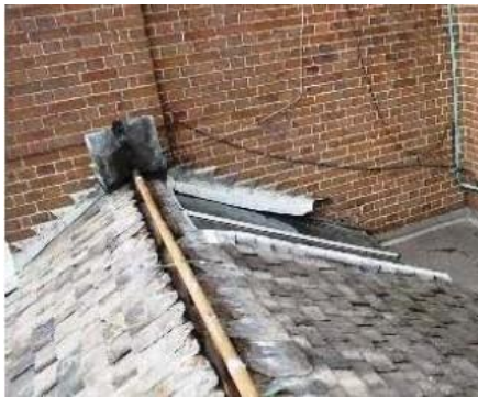
Stolen Lead Ridge and Flashings
