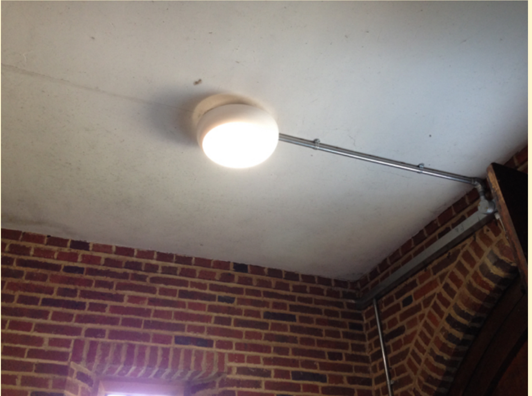
Porch lighting - LEDs which also serve as emergency lighting on battery (green dot indicates safety feature)
