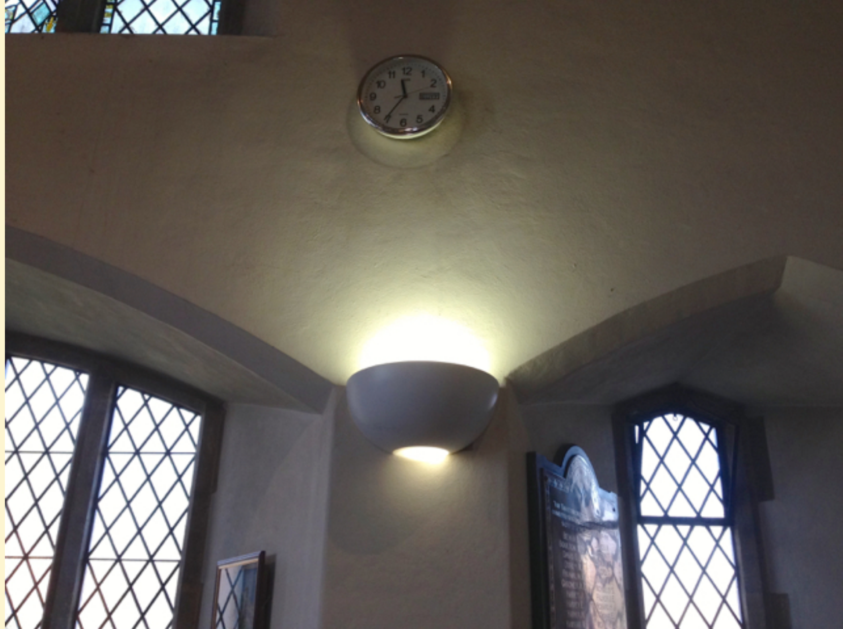
New LED lighting at West end of the nave provides both down-lighting and up-lighting
