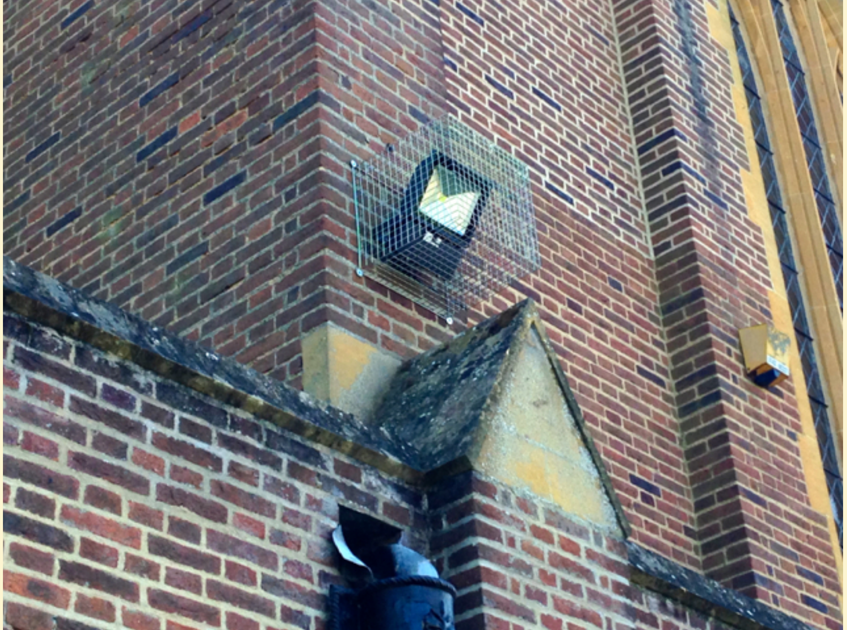
New LED floodlighting of car park automatically switches on and off at night-time in alignment with GMT and BST
