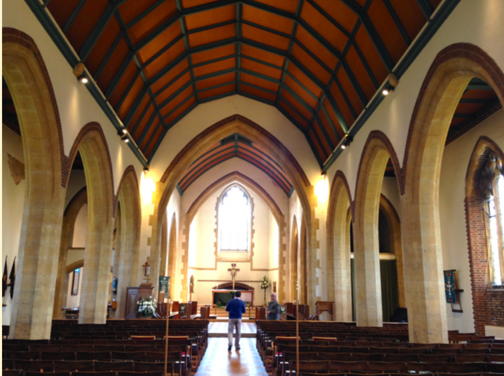
New LED lighting in the Nave has cables hidden in ceiling at minimal extra cost. Warmish lighting enhances the stone columns. Hardly any distracting glare.
