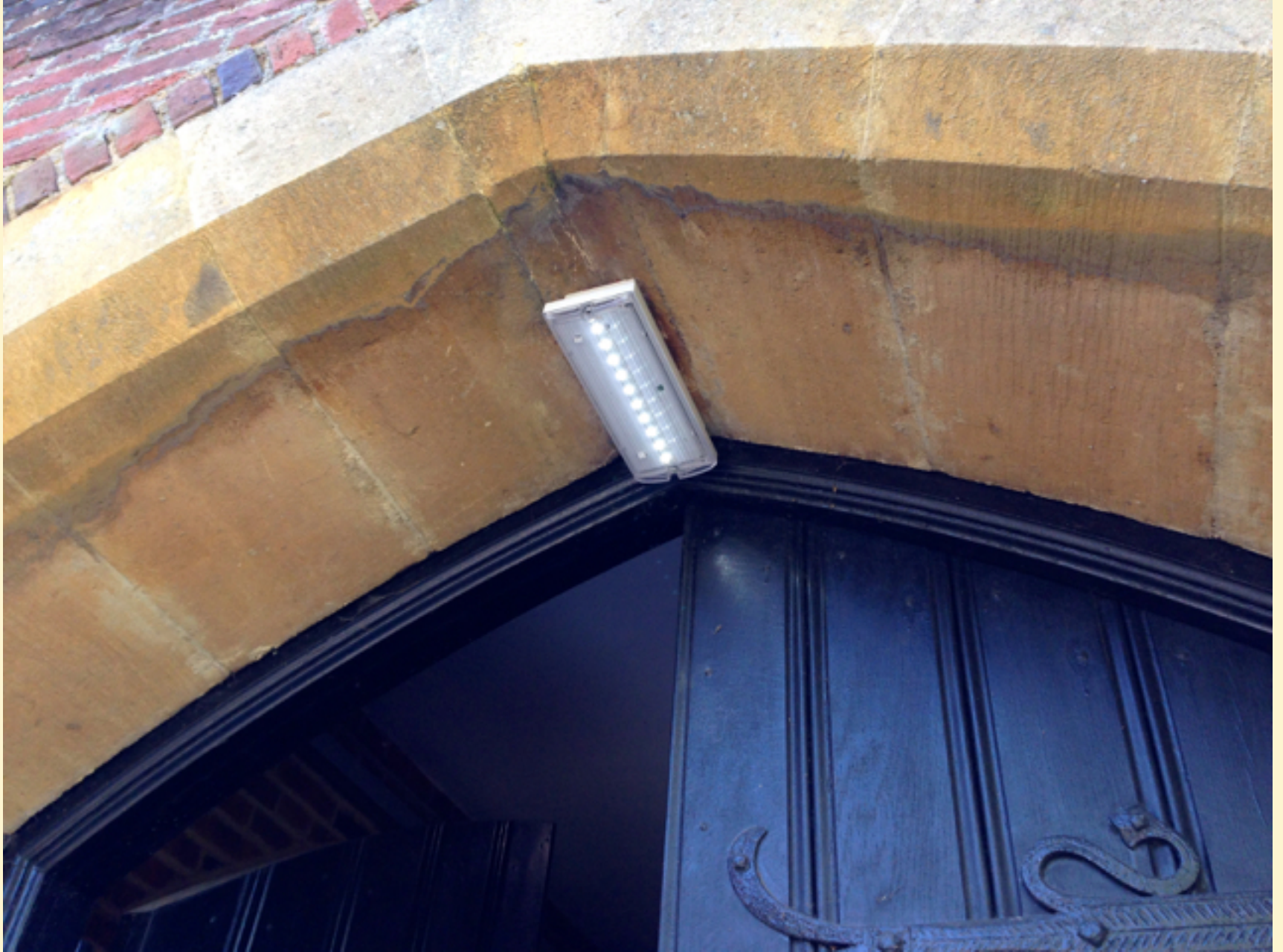
New LED lighting over the West Porch
