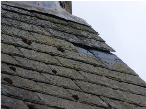
4. Nave North Slope. Missing verge slate at west end exposing nail heads. 4.1
