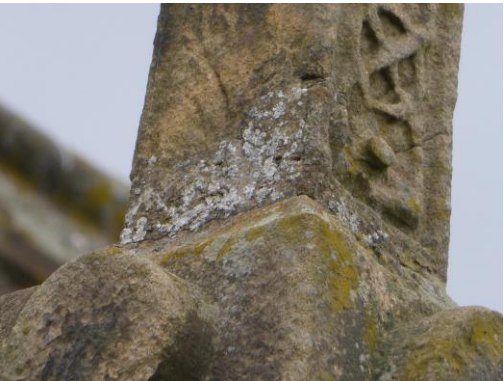
3. South Porch, South Gable. Possible cracks at base of finial cross. 3.2
