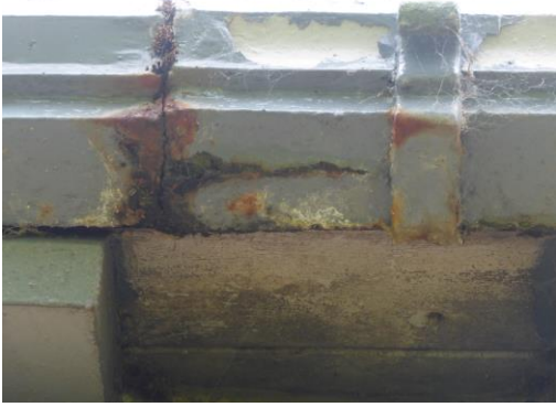
1. Nave North Wall. Cracked joint in gutter section. 3.2
