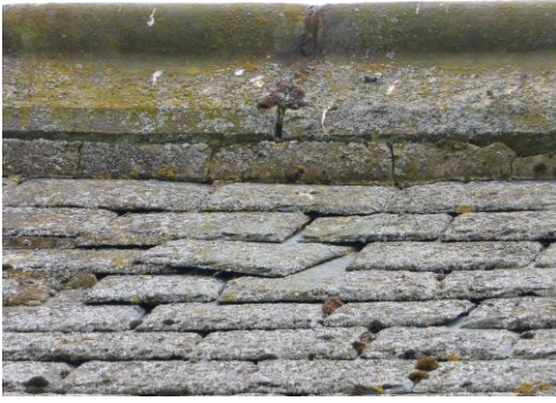
5. Chancel North Slope. Skewed slate near ridge. 4.2
