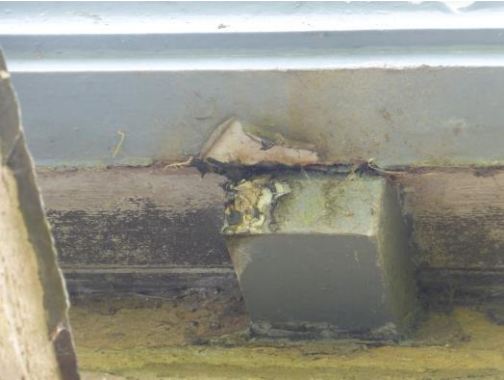
2. Nave North Wall. Blistering paint and rusting corner indicate a crack at the corner. 3.2
