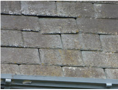
6. Chancel South Slope. Disturbed slate at bottom of slope. 4.5
