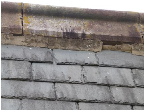
7. South Porch East Slope. Missing section of pointing at ridge tile. 4.7
