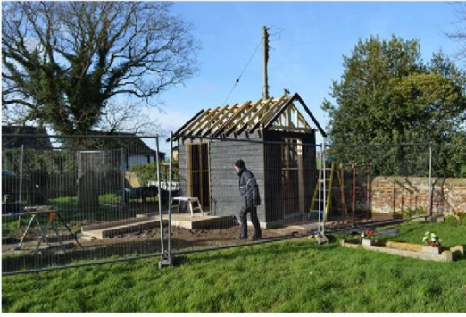
Left (Top and Middle): the Composting Toilet at Wickhampton, taking shape and finished.
