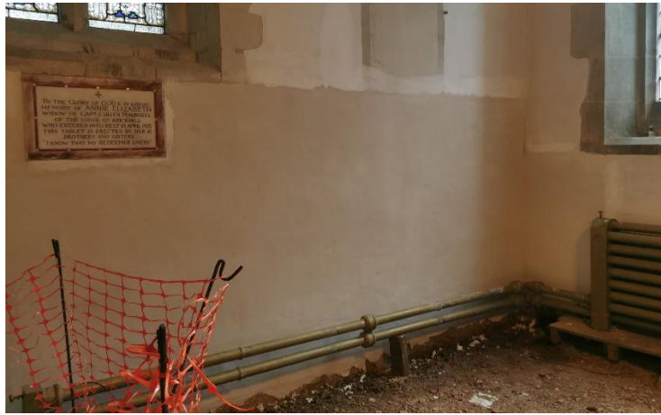
Work progressing in the church – wall re-plastered and floor ready for laying of slabs
