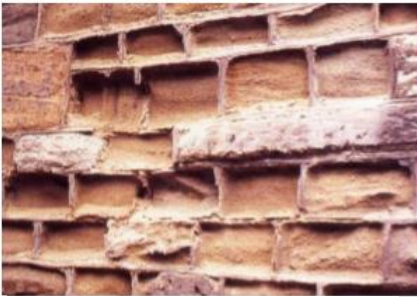
Hard cement pointing has caused the soft stone to decay
